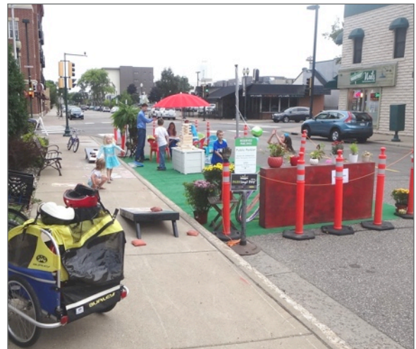
The City of Hopkins installed a temporary parklet downtown as part of Park(ing) Day 2014. The parklet was experiential and interactive, and helped residents and businesses think creatively about 8th Avenue. The City will install temporary streetscape and pedestrian and bicycle improvements along several blocks of 8th Avenue in 2015.
