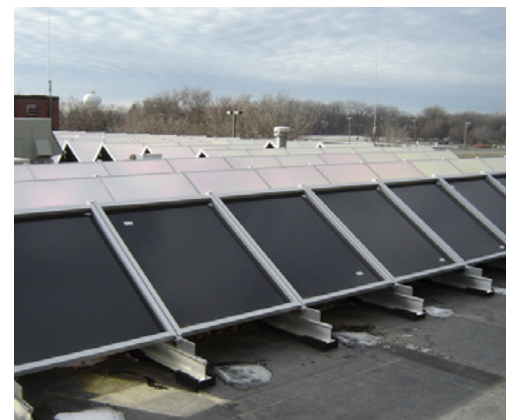
The City has a 40k open system through Dakota Electric supplementing the utility. The City initially leased the panels and will own them in the future.
