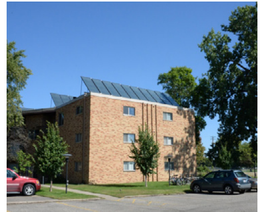
Solar panels are on the roof an apartment complex at Fairview and Larpenteur in Falcon Heights: Within the City there are solar installations on single-family, multi-family, and City-owned buildings.
