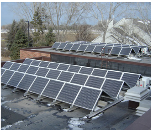
In 2012, Falcon Heights had solar panels installed on the roof of the City Hall. Solar power now account for 40-60% of City Hall power.
