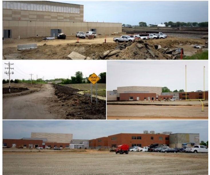
Construction photos of Clearwater Middle School transition and expansion into the new Waconia High School. The left photo in the middle row illustrates the expansion of CSAH 10 and a new roundabout that will create better access to roads and the school.
