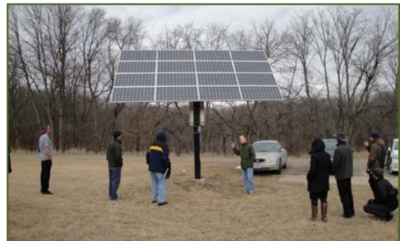
Ground Mount System, CERTs
