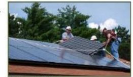
Rooftop Solar, MREA
