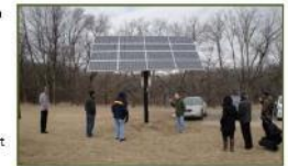
Ground Mount System, CERTS
