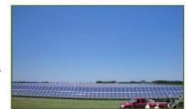
Solar Farm, CERTS
