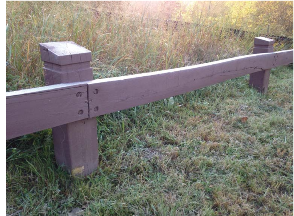
TIMBER ACCESS CONTROL AT PARKING LOT EDGE
