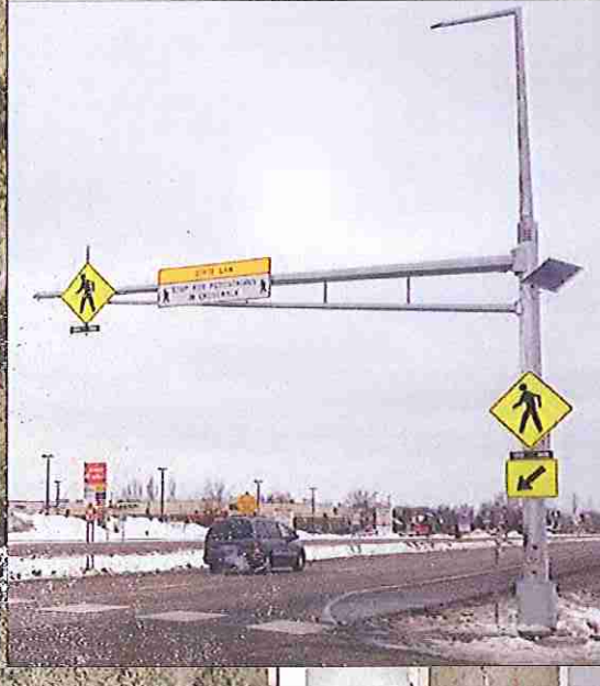
MAST ARM MOUNTED RRFB
