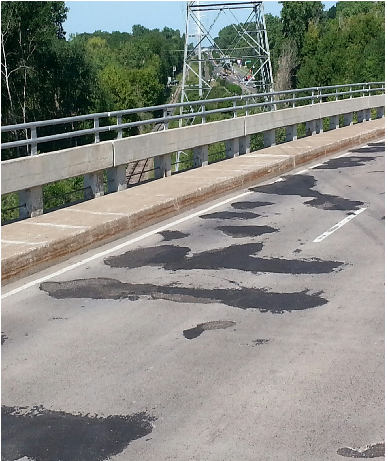
Bridge 62519 Deck Condition
