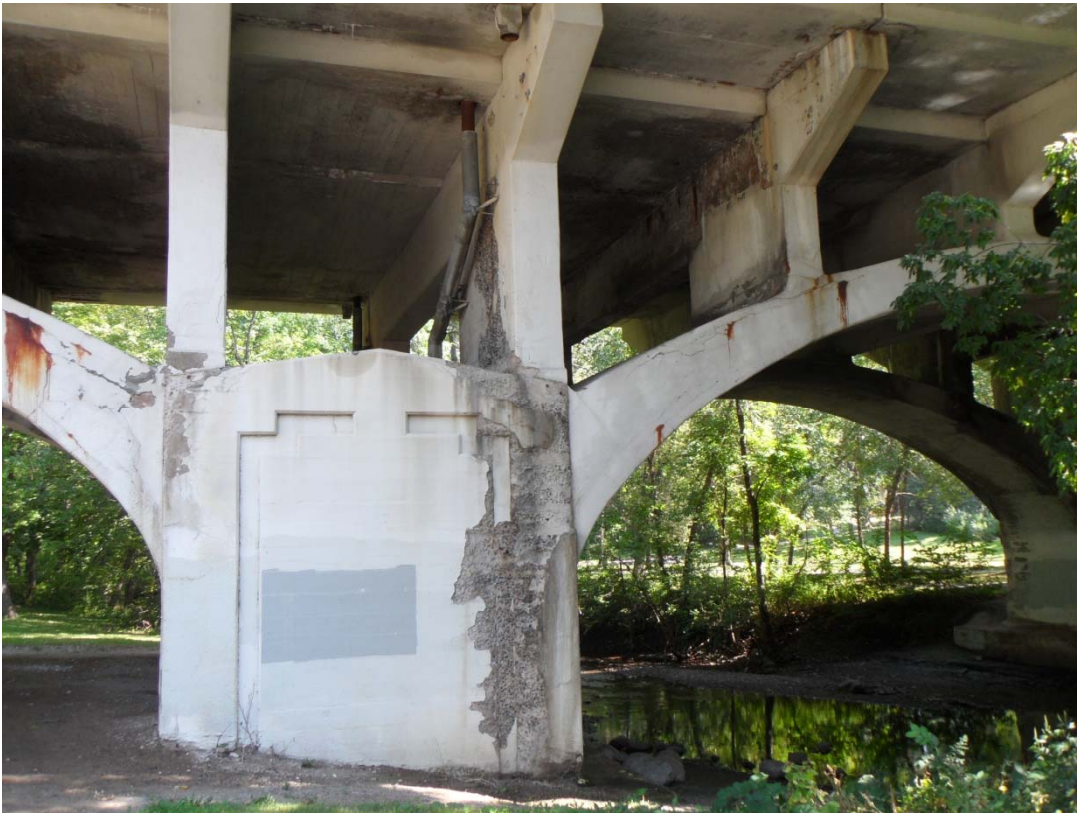
Figure 4: Spall on Pier at Downspout Location
