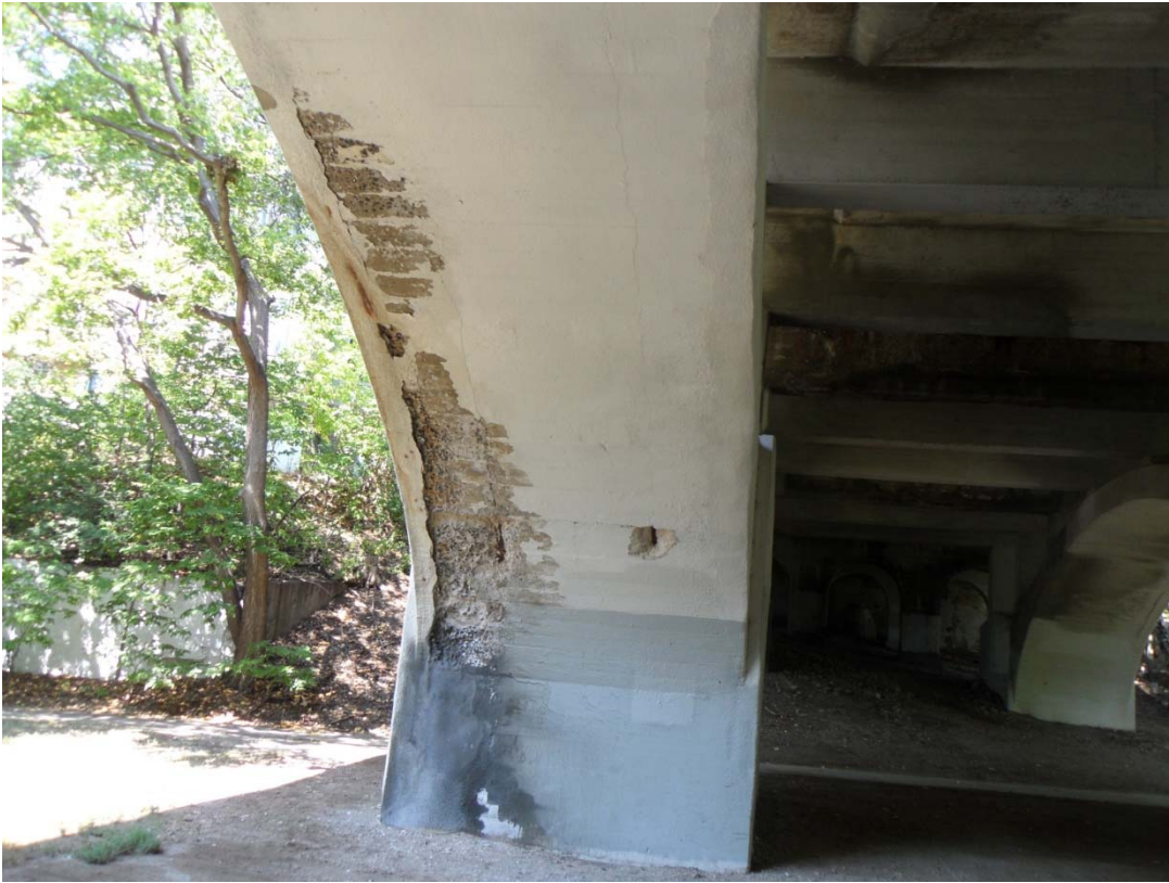
Figure 3: Spalls on Arch
