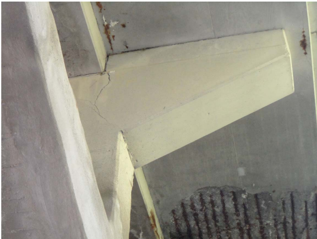
Figure 10: Crack on Cantilever Bracket
