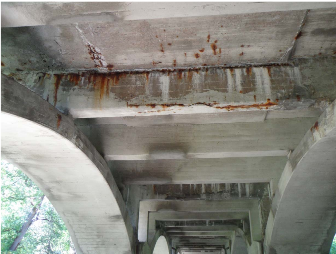
Figure 8: Previous Floorbeam Repair with Rust Seeping Through
