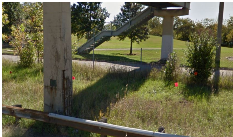
Figure 4: Existing Column Damage
