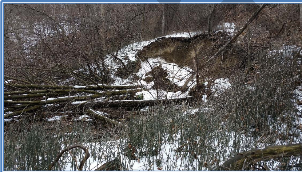
Photograph 19 Northeast Toe Damage
