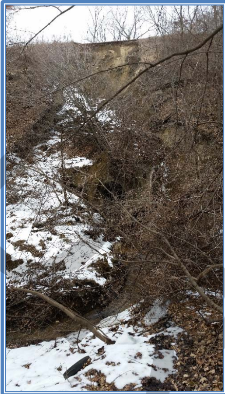
Photograph 7 South Pipe Crossing Damage (looking up-slope from toe)
