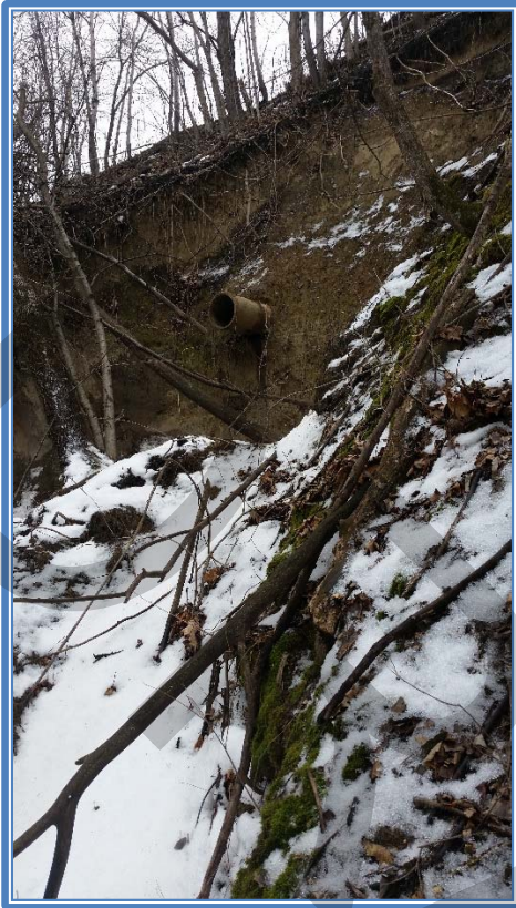
Photograph 13 North Pipe Crossing Damage (looking up-slope from toe)
