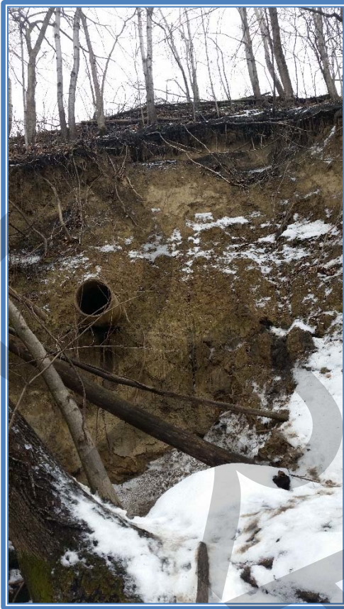
Photograph 15 North Pipe Crossing Damage (looking up-slope from toe)
