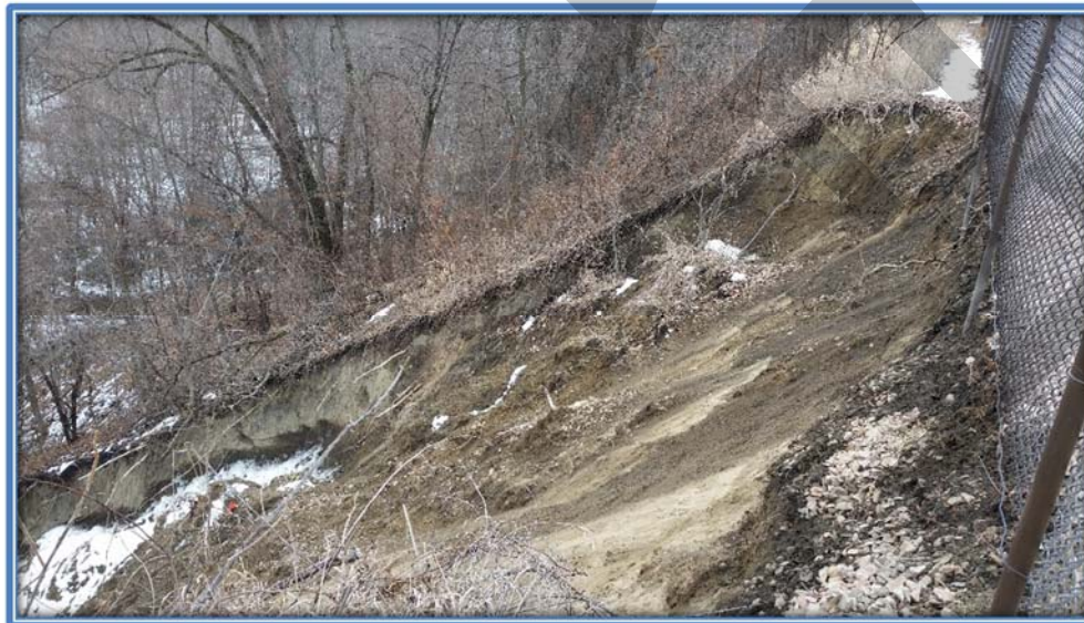
Photograph 2 South Pipe Crossing Damage (looking down-slope from trail)
