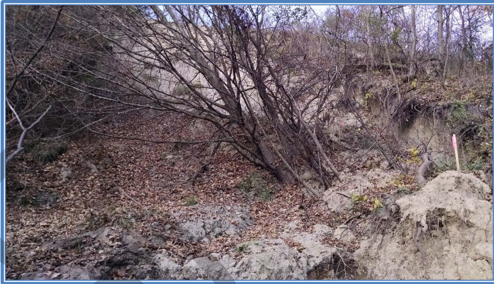
Photograph 9 South Pipe Crossing Damage (looking up-slope from toe)
