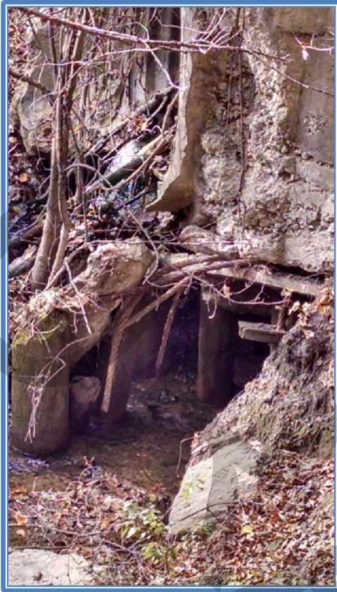
Photograph 5 South Pipe Crossing Damage (headwall damage)
