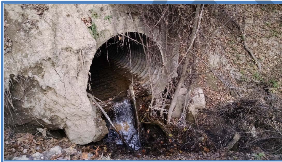
Photograph 6 South Pipe Crossing Damage (CMP exiting toe of slope)
