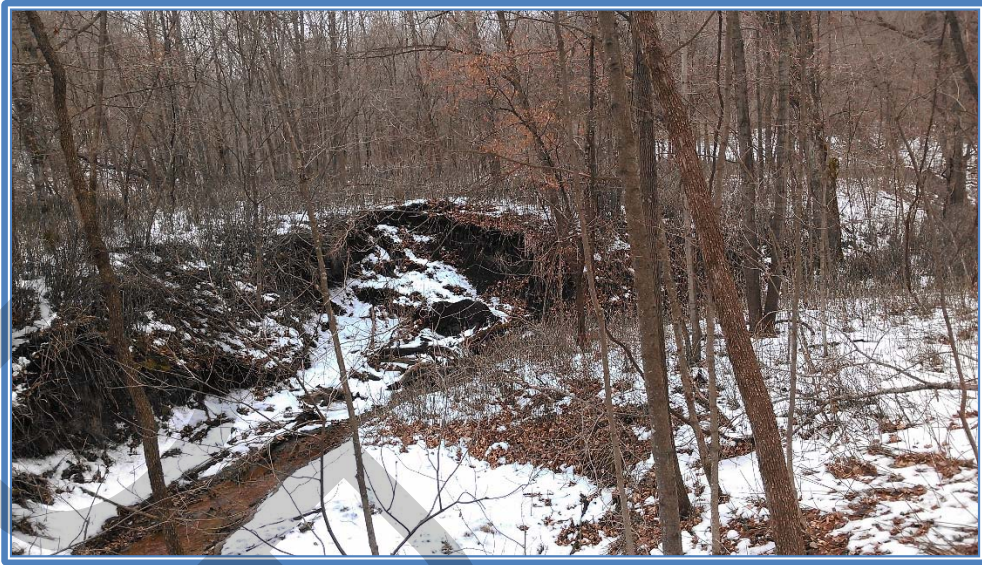
Photograph 20 Southwest Toe Damage
