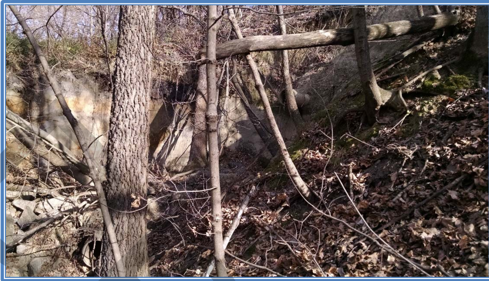
Photograph 17 North Pipe Crossing Damage (looking up-slope from toe)
