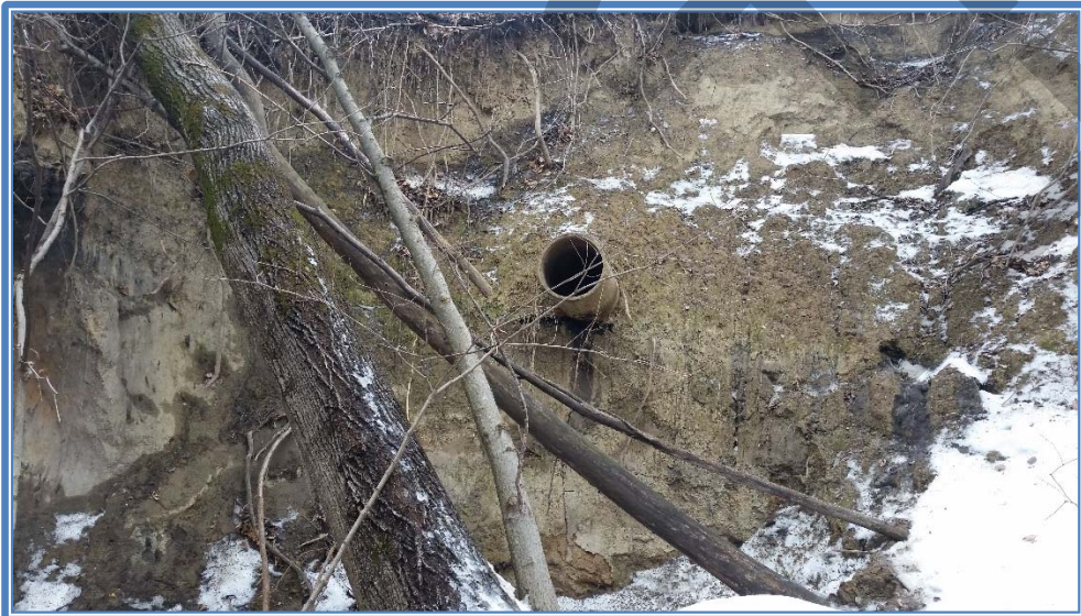
Photograph 16 North Pipe Crossing Damage (looking up-slope from toe)
