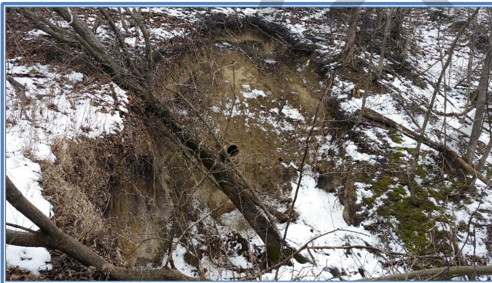
Photograph 14 North Pipe Crossing Damage (looking down from side slope)
