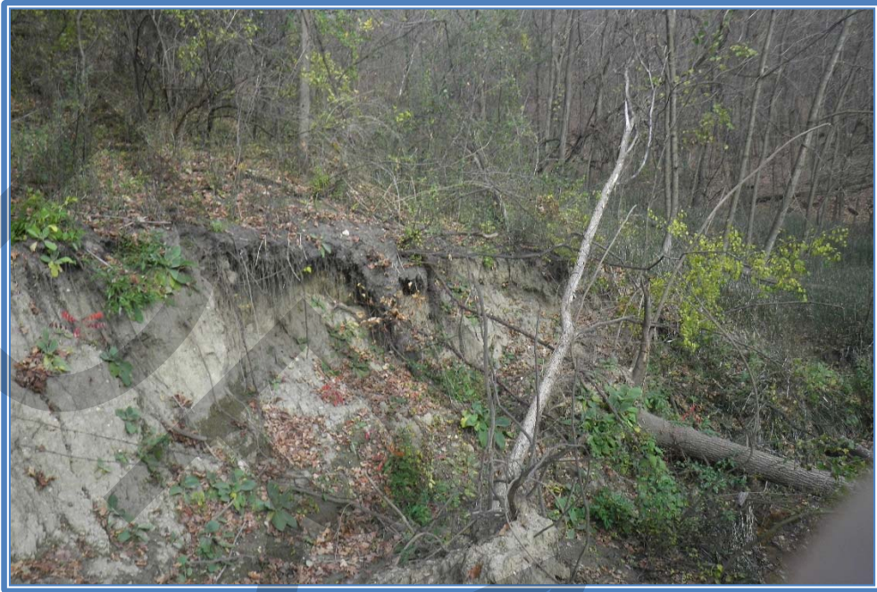
Photograph 18 Northeast Toe Damage
