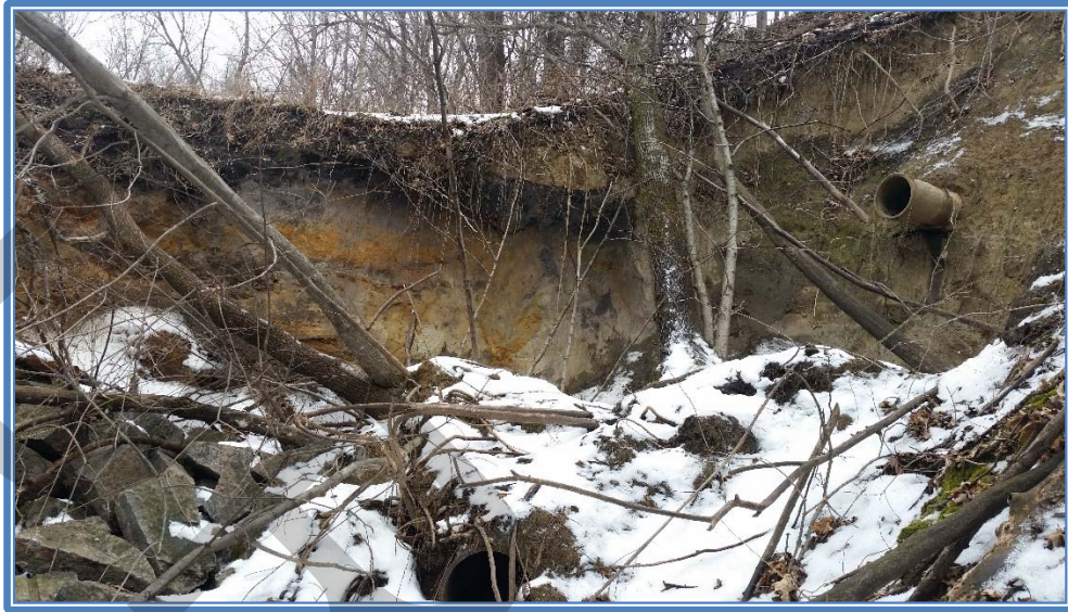
Photograph 11 North Pipe Crossing Damage (looking up-slope from toe)
