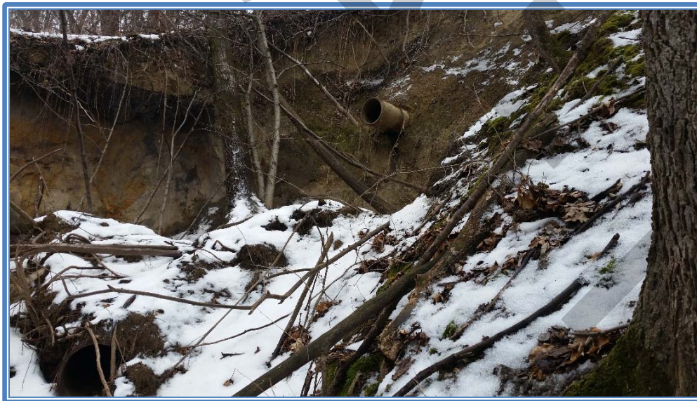
Photograph 12 North Pipe Crossing Damage (looking up-slope from toe)
