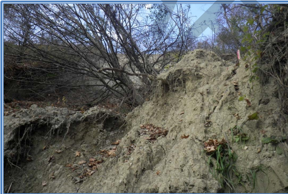
Photograph 8 South Pipe Crossing Damage (looking up-slope from toe)
