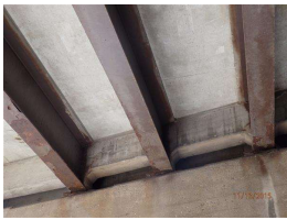
1. beam ends pier 1 - rusty - north face.JPG
