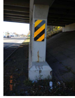
7. column S.side damage_1.jpg
