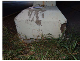
28. Impact damage at base of W end of Pier 2.JPG
