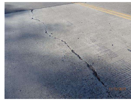
4. longitudinal cracks south approach panel.JPG
