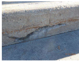
3. longitudinal cracking at curb face east side mid span.JPG
