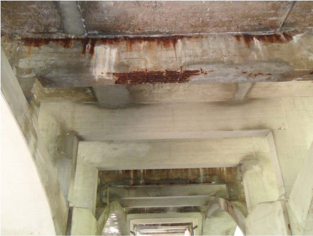
Figure 7: Floorbeam Spall Adjacent to Previous Repair
