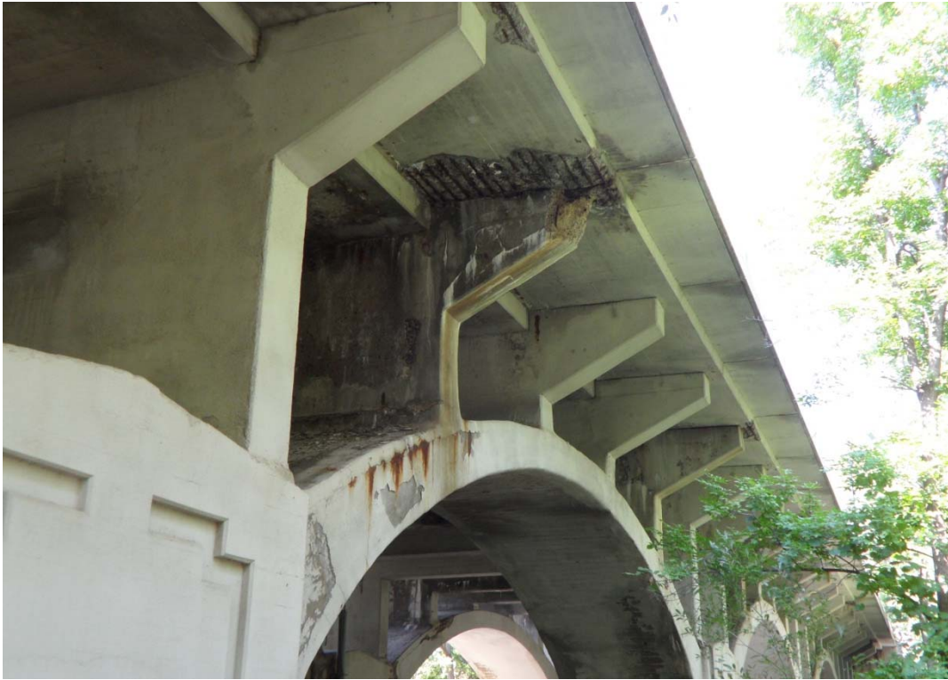
Figure 5: Spalls and Cracks on All Elements
