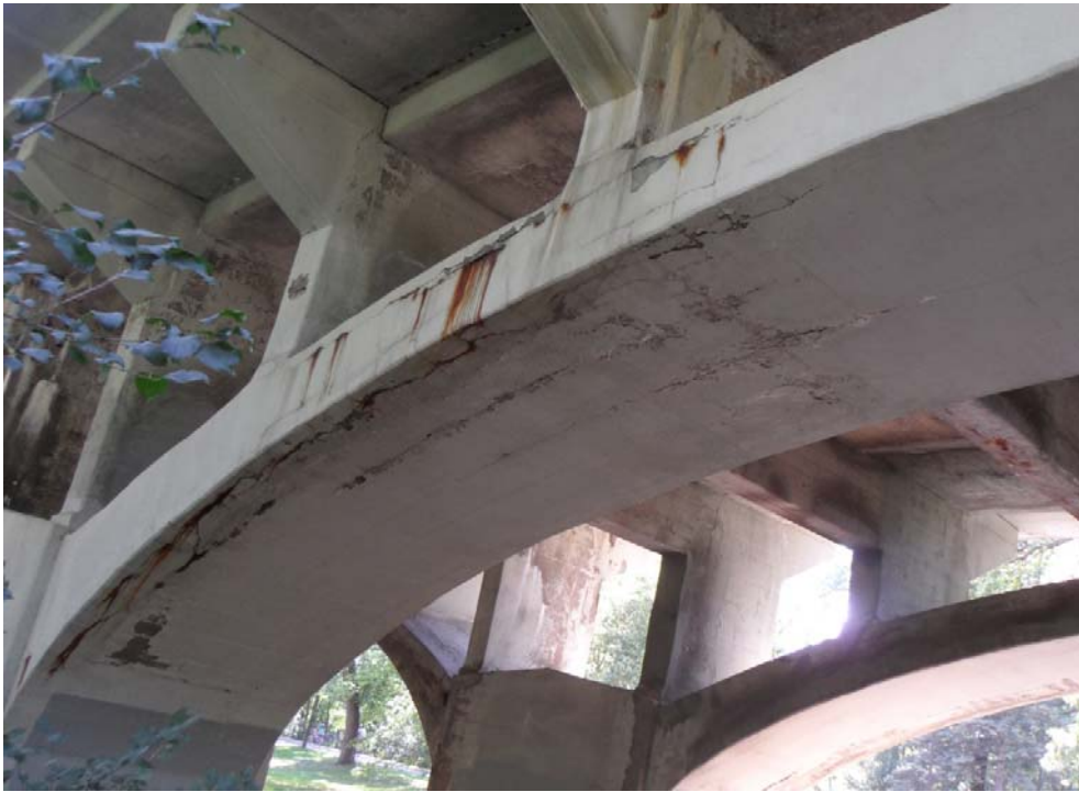
Figure 2: Cracks on Arch
