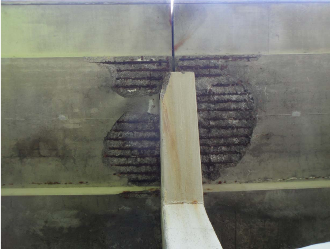
Figure 9: Spall on Underside of Deck
