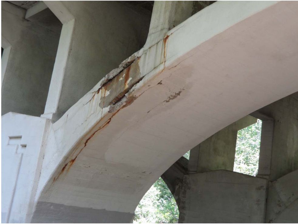
Figure 1: Major Crack on Arch
