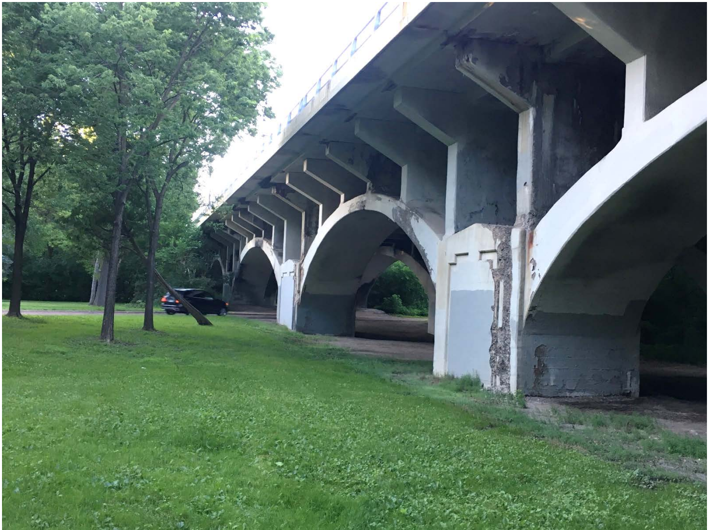
Existing Condition - Nicollet Ave. South Bridge over Minnehaha Creek
