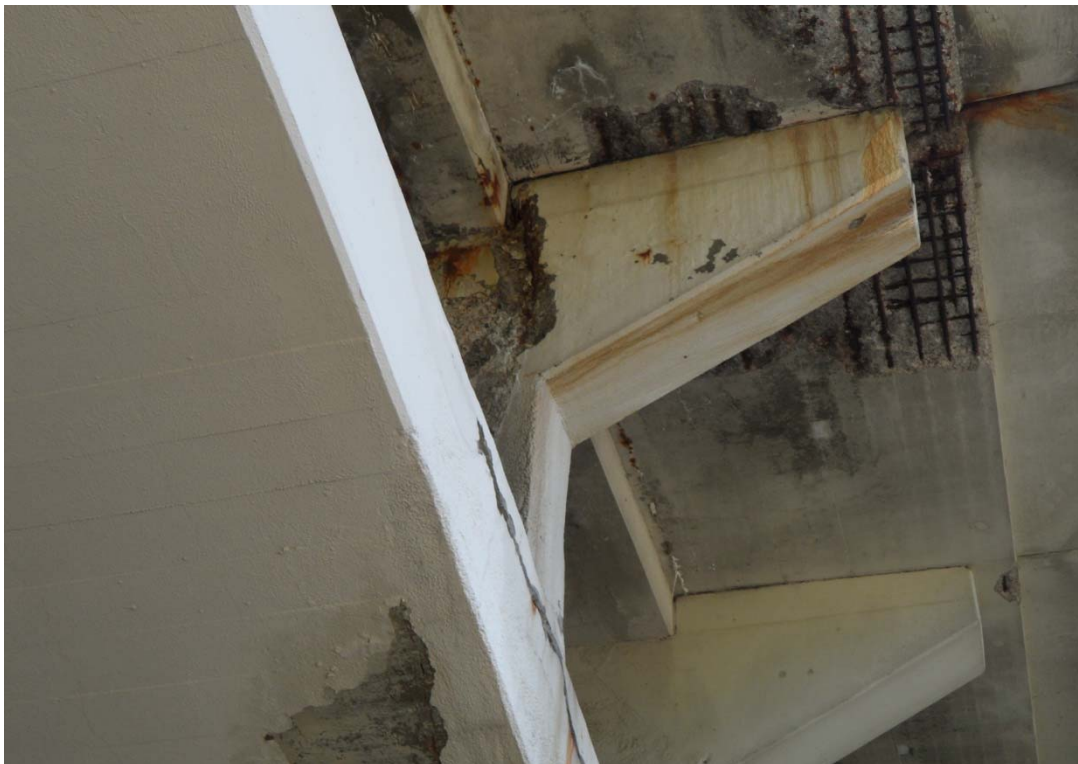
Figure 6: Spall on Spandrel Column and Cantilever Bracket
