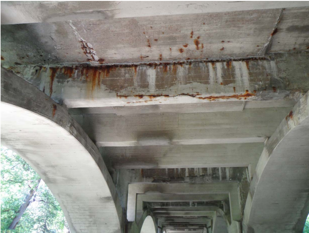
Figure 8: Previous Floorbeam Repair with Rust Seeping Through
