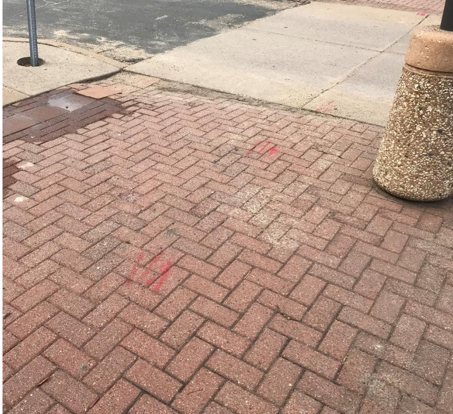
Existing sidewalks are aging and crumbling, limiting accessibility and detracting from user experience.
