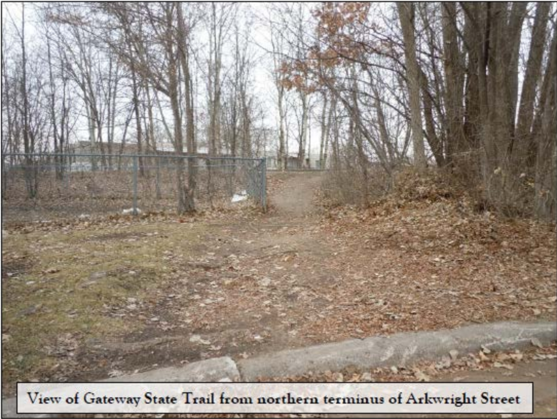
Project Component 3: Existing dirt path connecting Arkwright St. to the Gateway State Trail.
