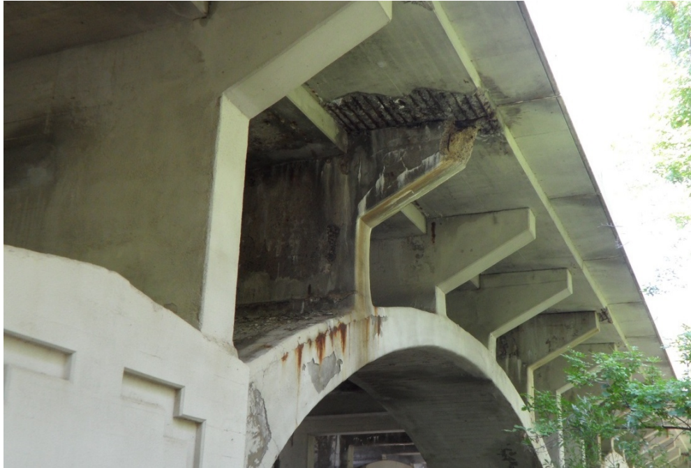
Figure 10: Concrete Spalls and Cracks on all Elements
