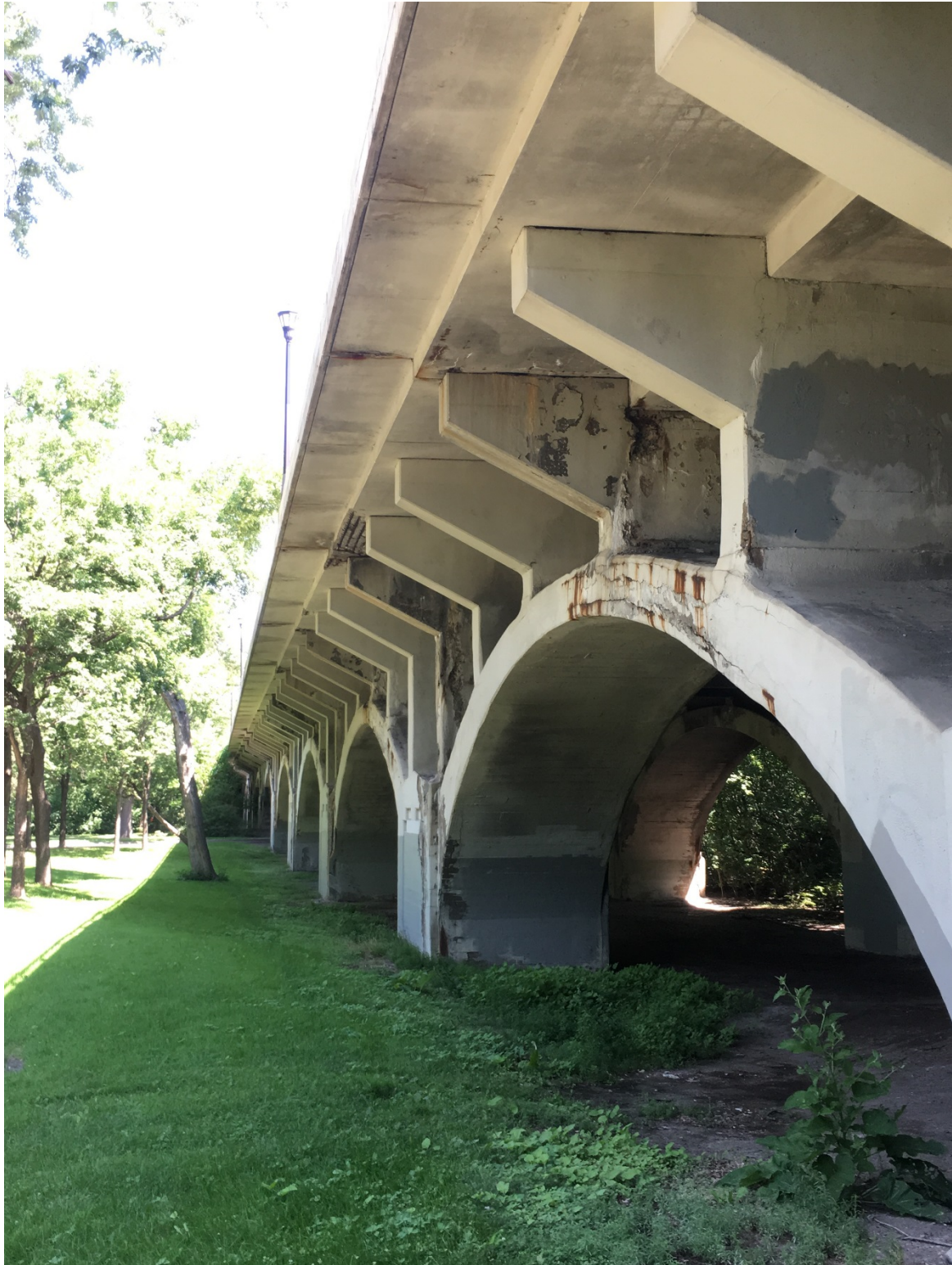
Existing Condition - Nicollet Ave. South Bridge over Minnehaha Creek
