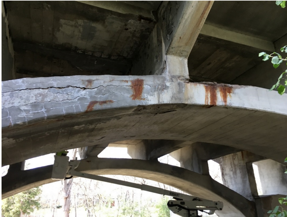
Figure 2: Major Crack and Concrete Deterioration on Arch Rib
