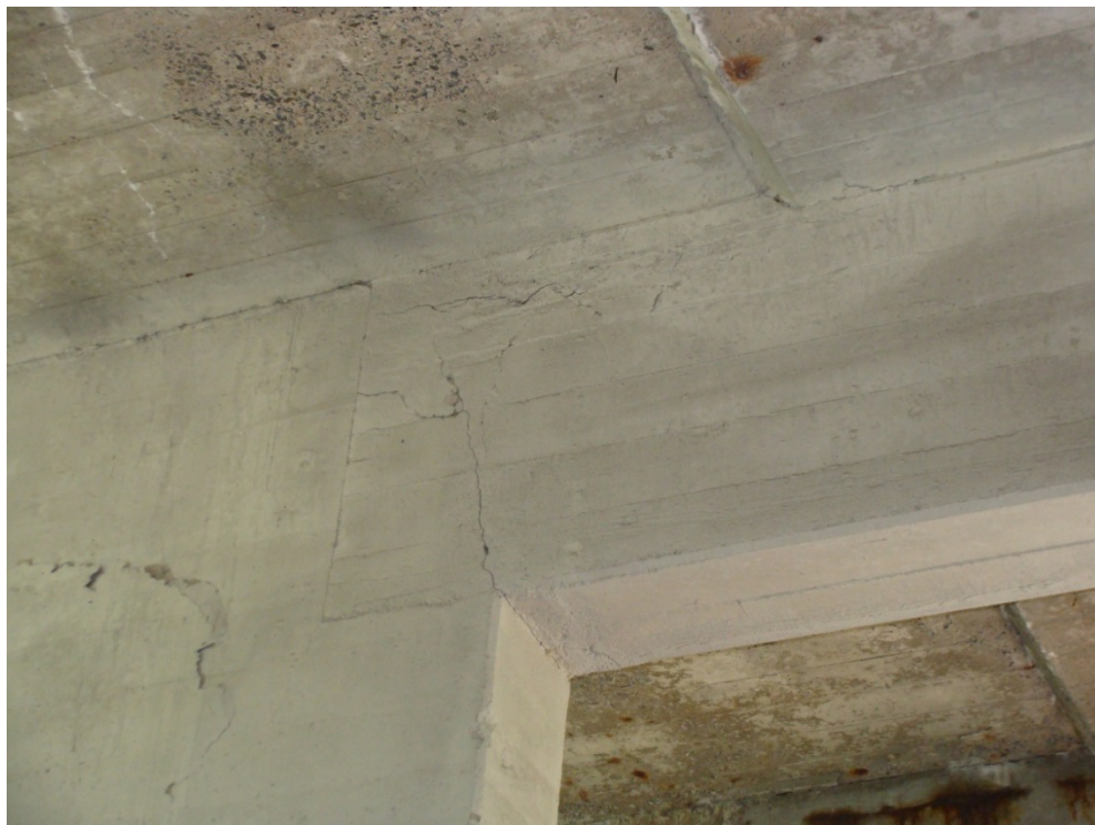
Figure 13: Crack on Floorbeam
