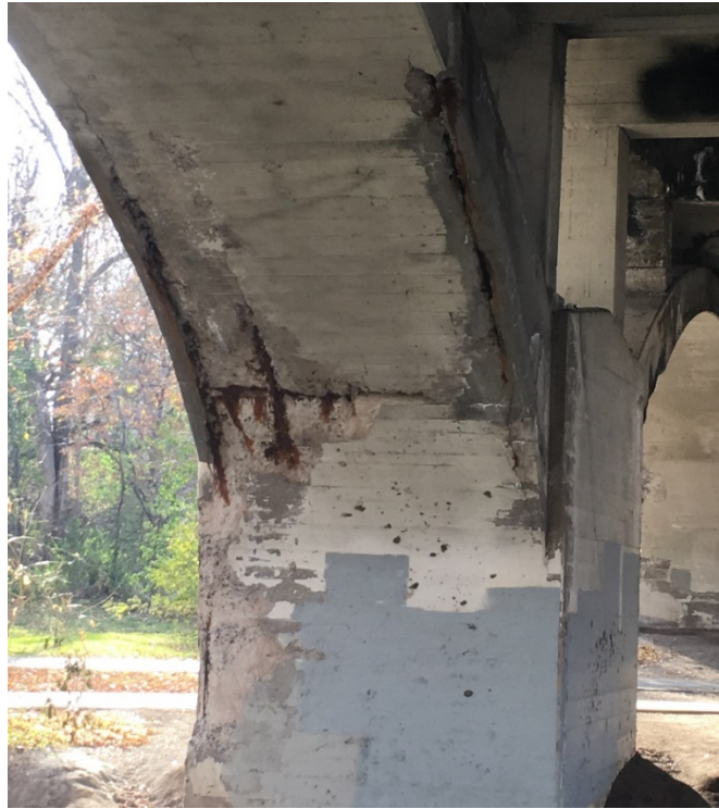
Figure 8: Pier Delaminated Concrete with Exposed Reinforcement
