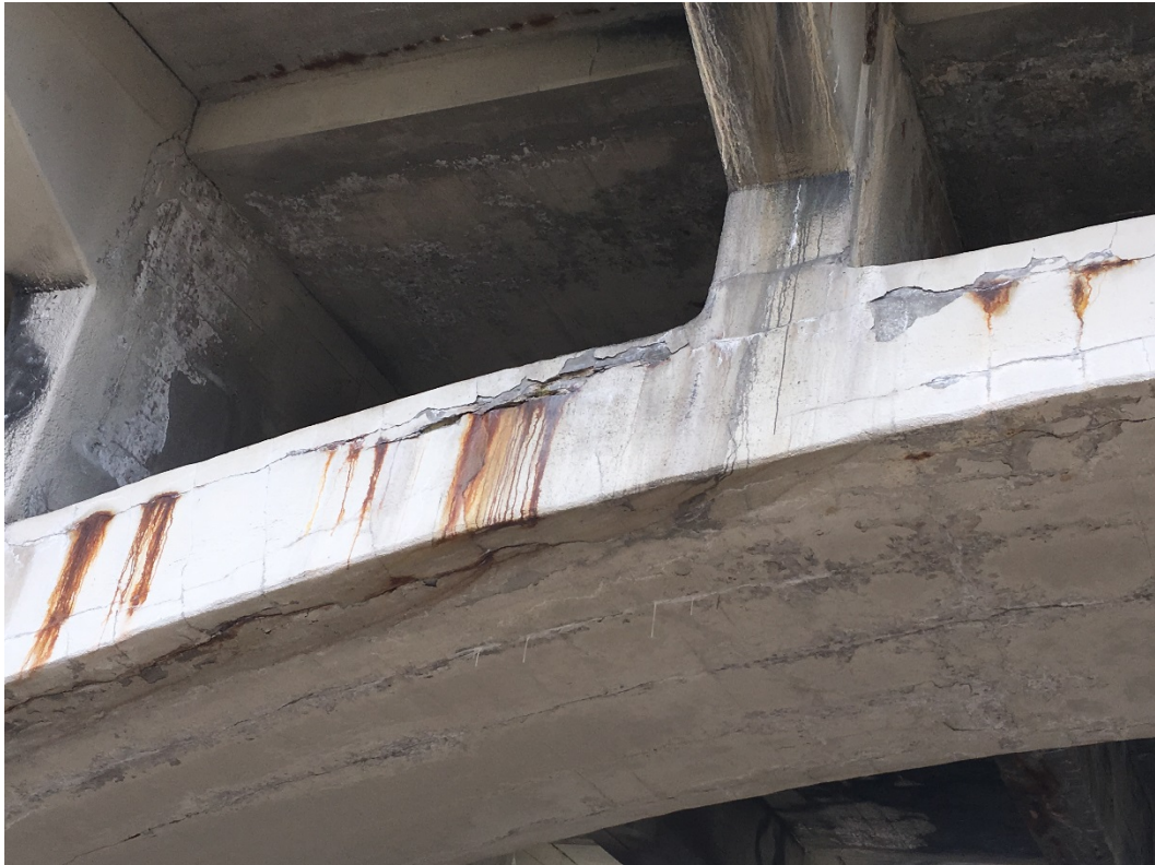
Figure 4: Cracks on Arch Rib
