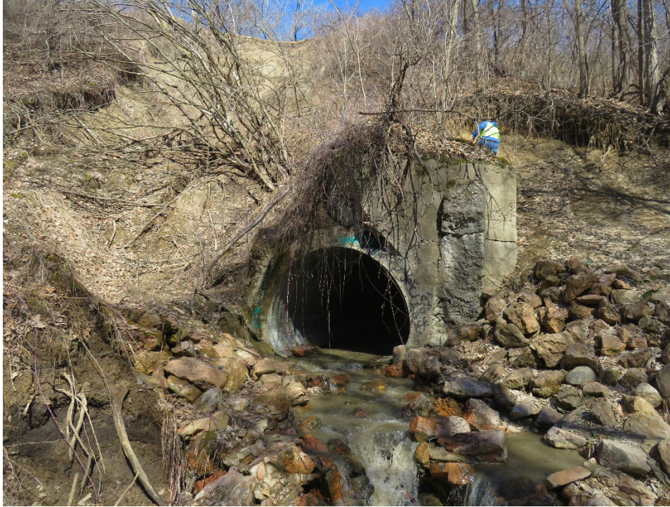
Figure 4 – Slope failure area at the base of the trail where a large culvert is located. The trail is approximately 80 feet above the culvert invert elevation.
