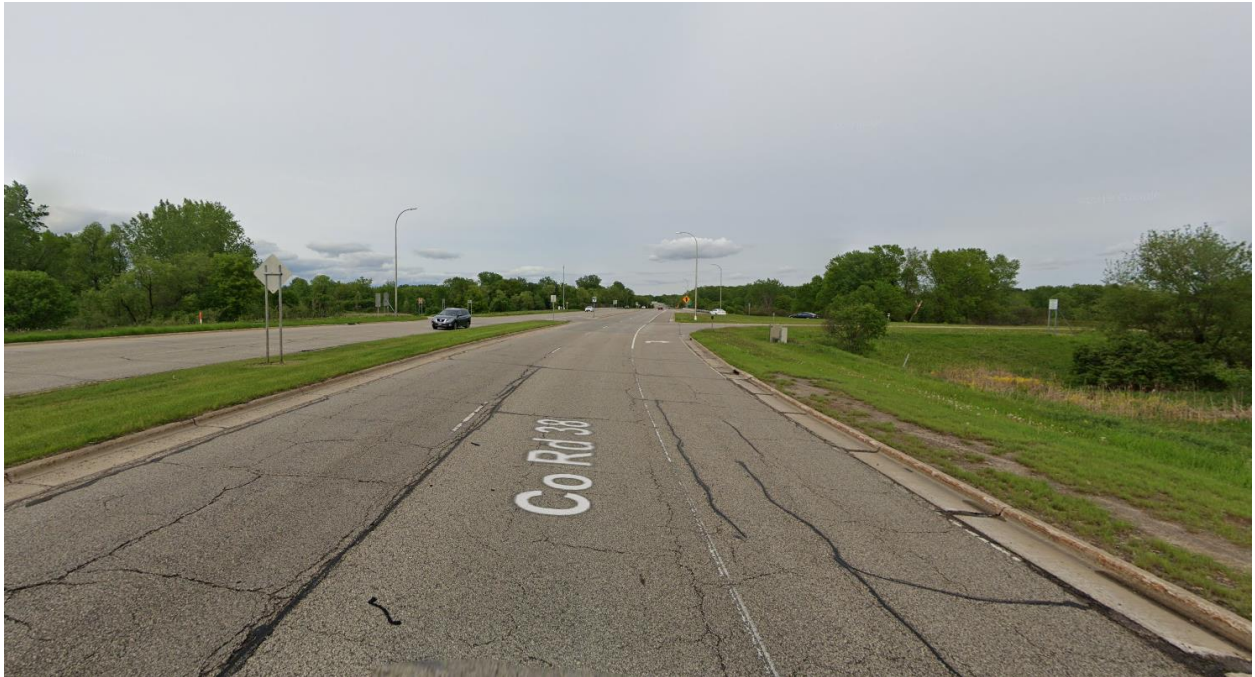
Existing Conditions: CSAH 38 westbound, approaching Cedar Avenue (TH77) intersection; no shoulder facilities.
