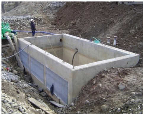
Figure 20. Water Meter Vault
