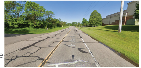
Hudson Road has no safe ped/bike access
