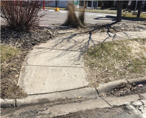
Project Location #18, example of existing pedestrian curb ramp in need of replacement to comply with ADA standards
