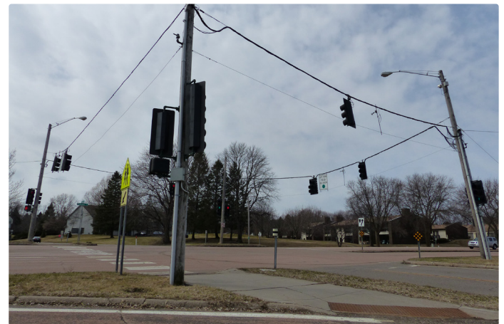
Existing Carver County Traffic Signal
