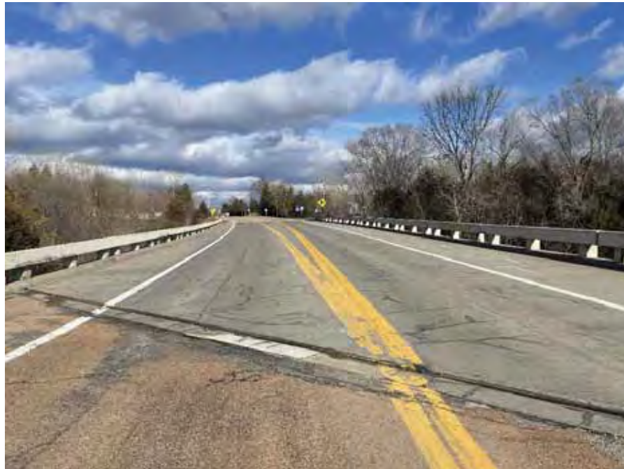
Existing roadway surface, demonstrating cracks and a lack of pedestrian or bicycle facilities
