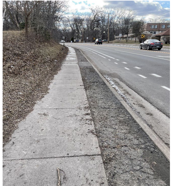
Degrading sidewalk and paved boulevard assets, south side of Bass Lake Rd.
