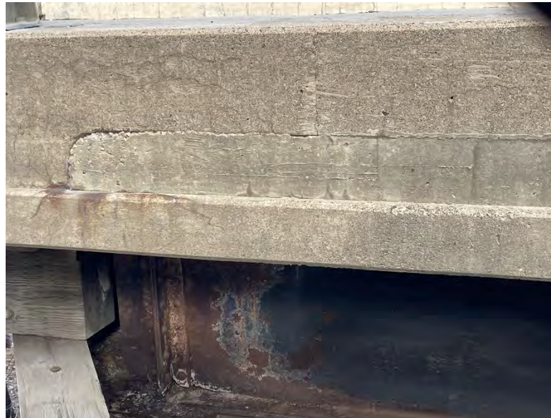
Cracks in the concrete along the existing bridge railing.
