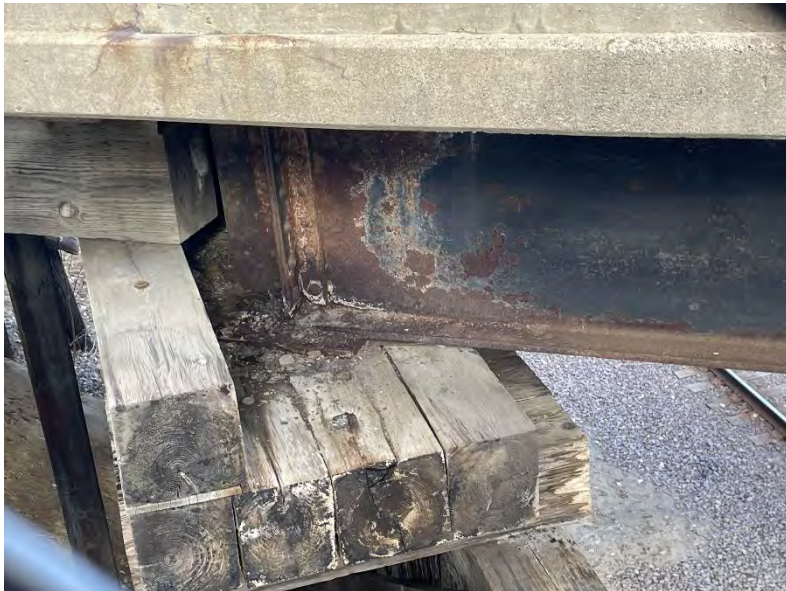
View of the top of an aging timber pier, including rusting along the steel beam span.
