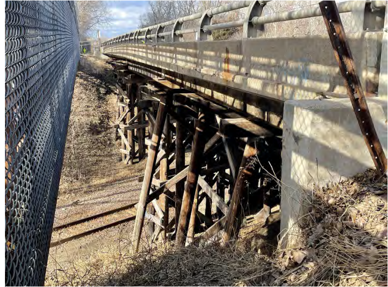
View of the functionally obsolete timber bridge span and piers over the Twin Cities & Western Railroad.
