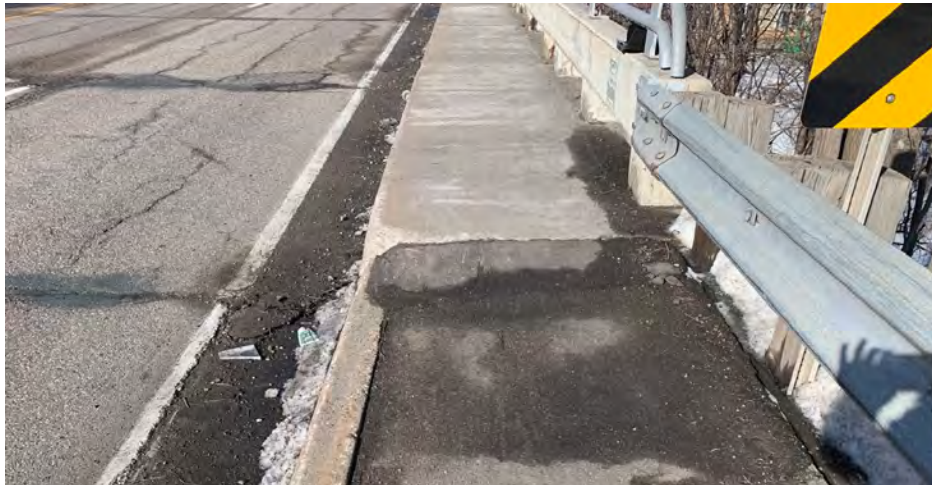
Existing Deteriorated Bridge Sidewalk
