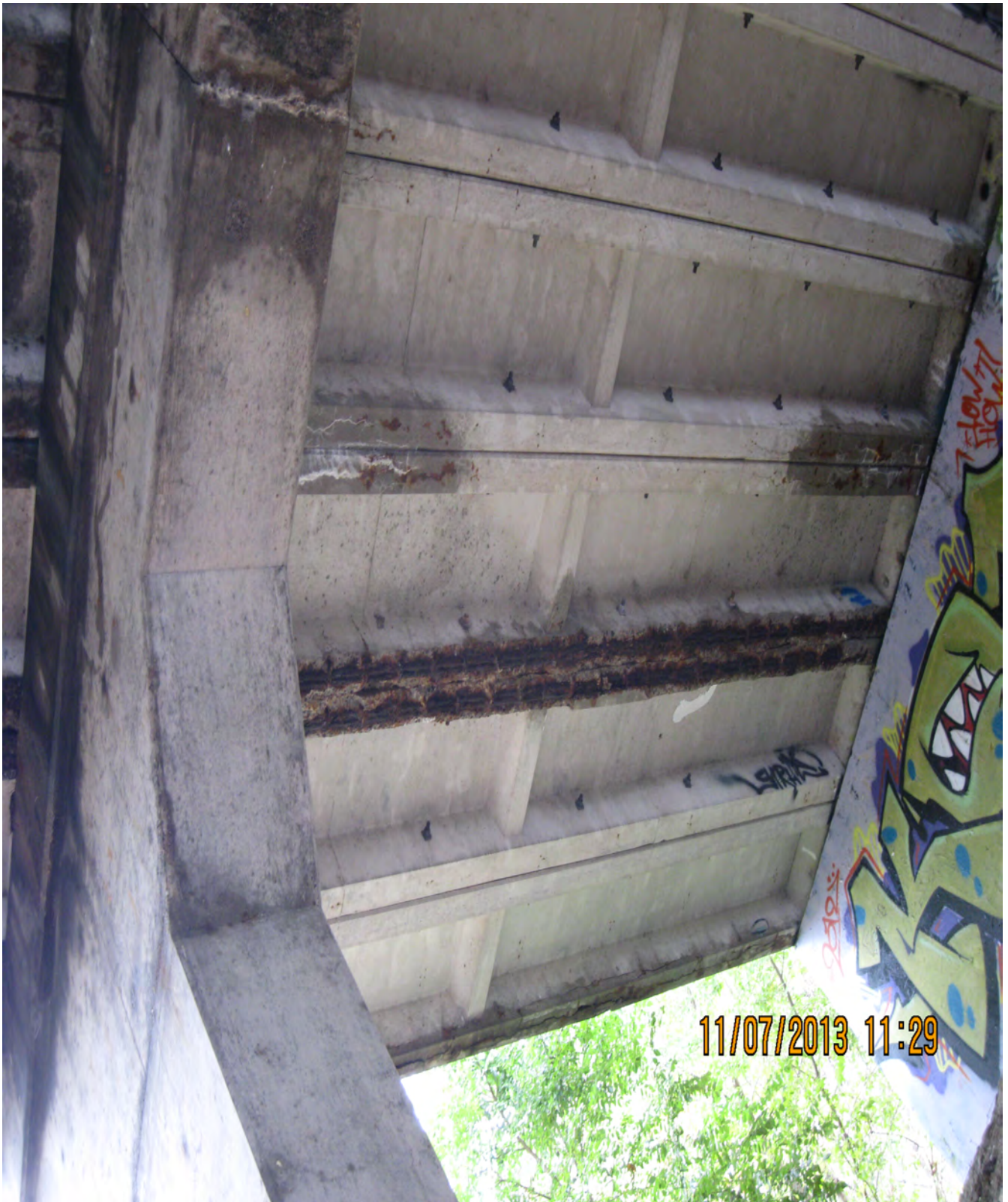
West Span, Bridge 4533, showing beam spalling and delamination
