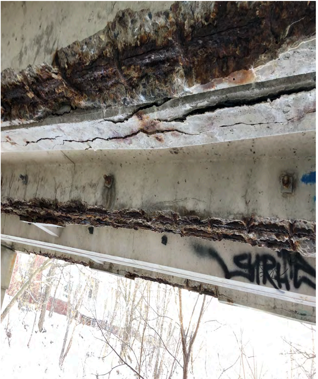
Bridge 4533 beam condition showing section loss
