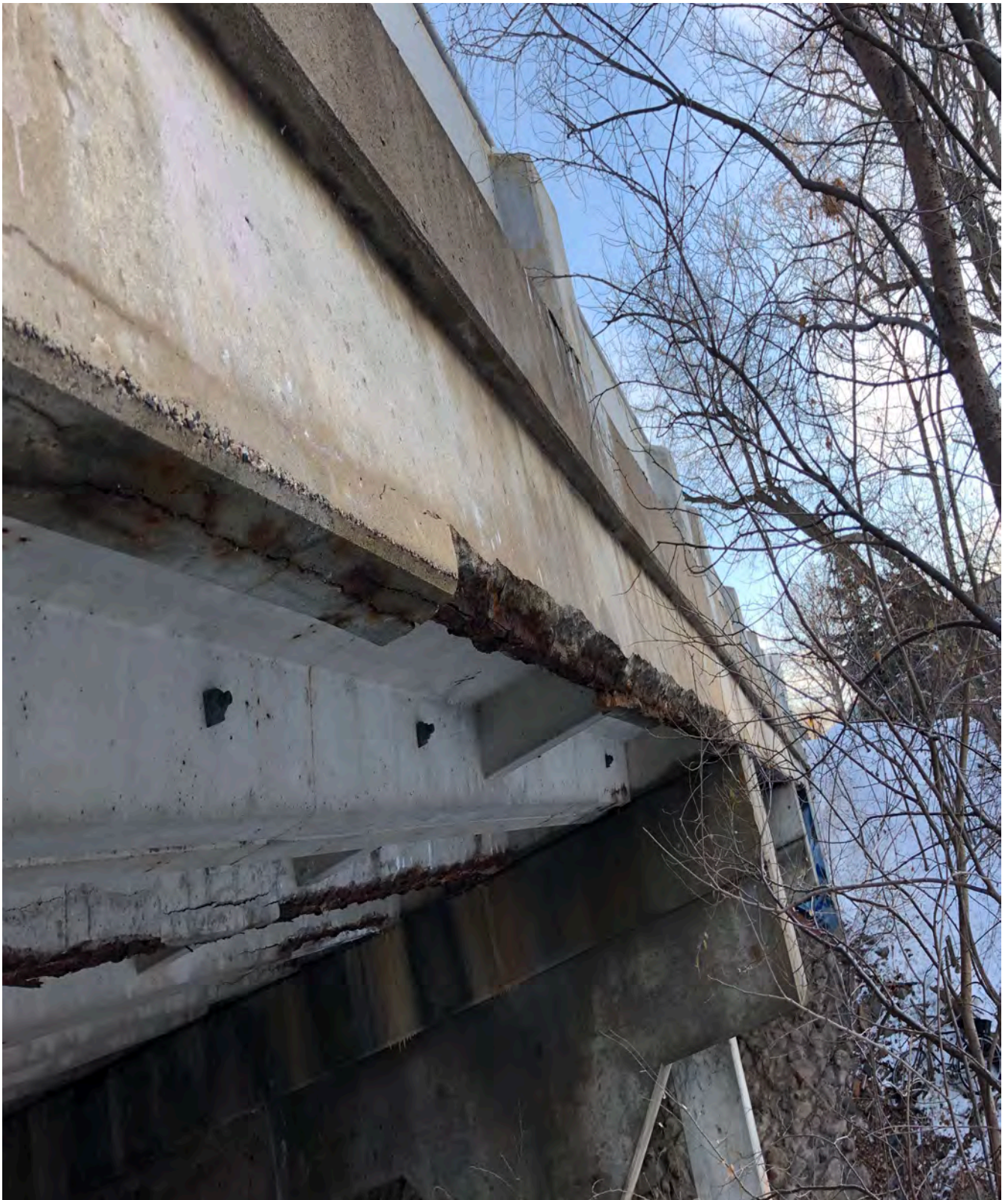
Bridge 4533 exterior beam showing section loss
