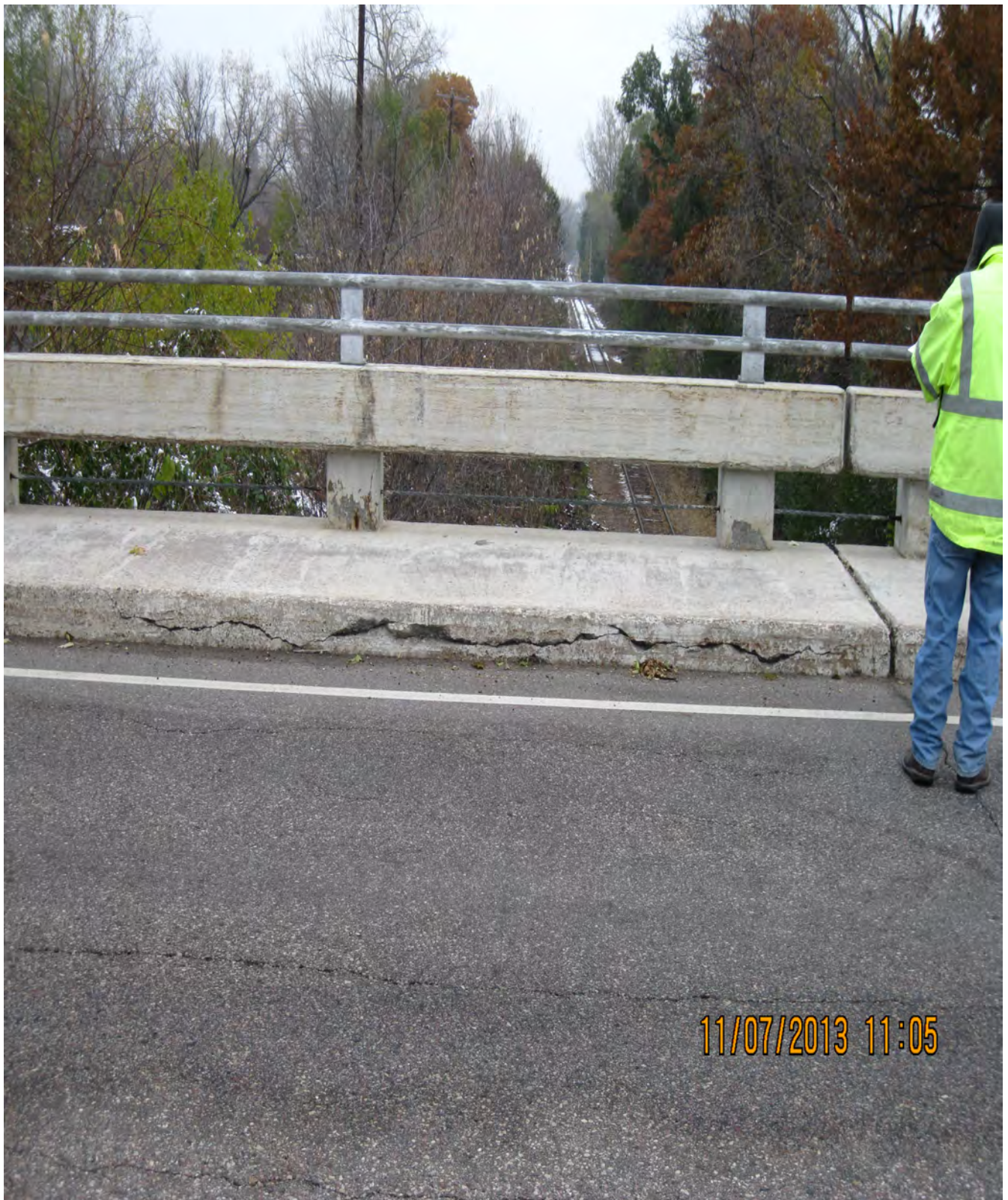
Crack and deterioration of north curb.
