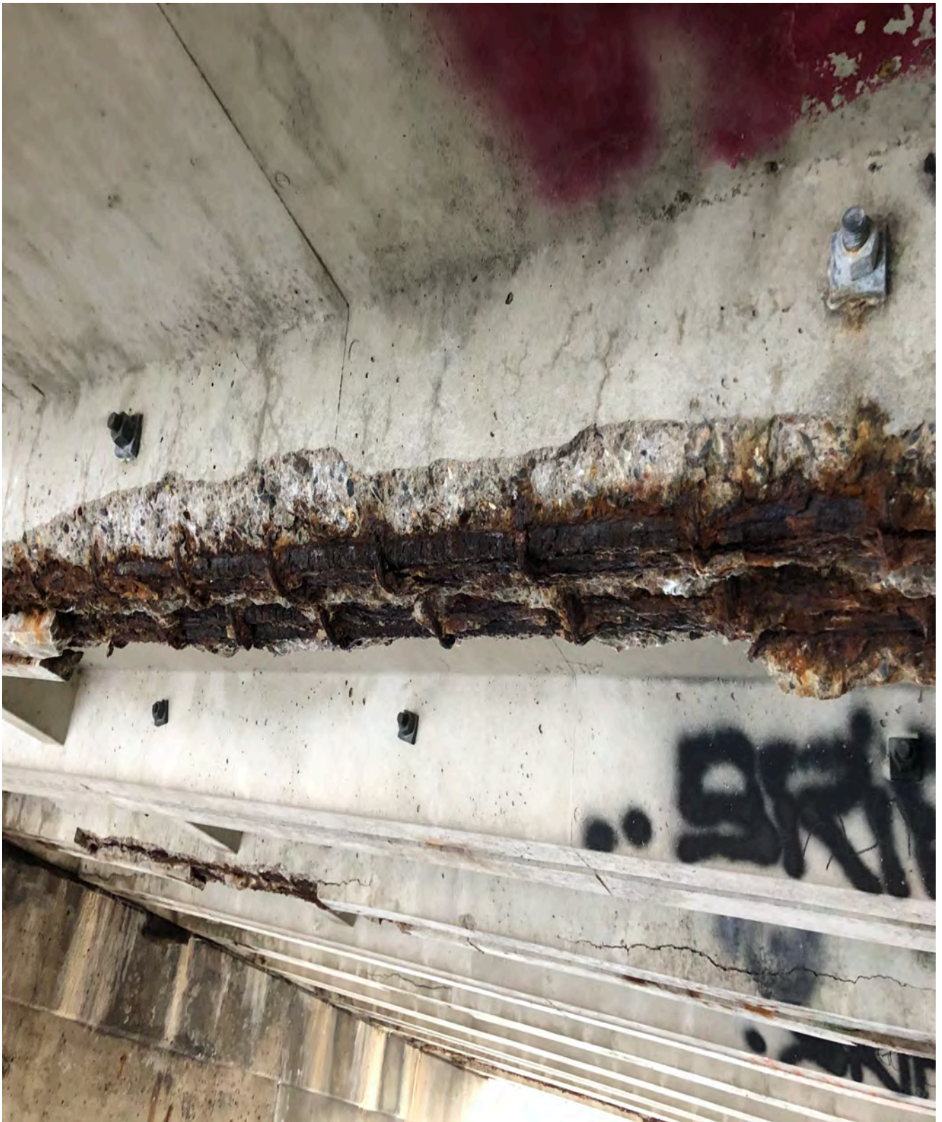
Bridge 4533 beam condition showing section loss
