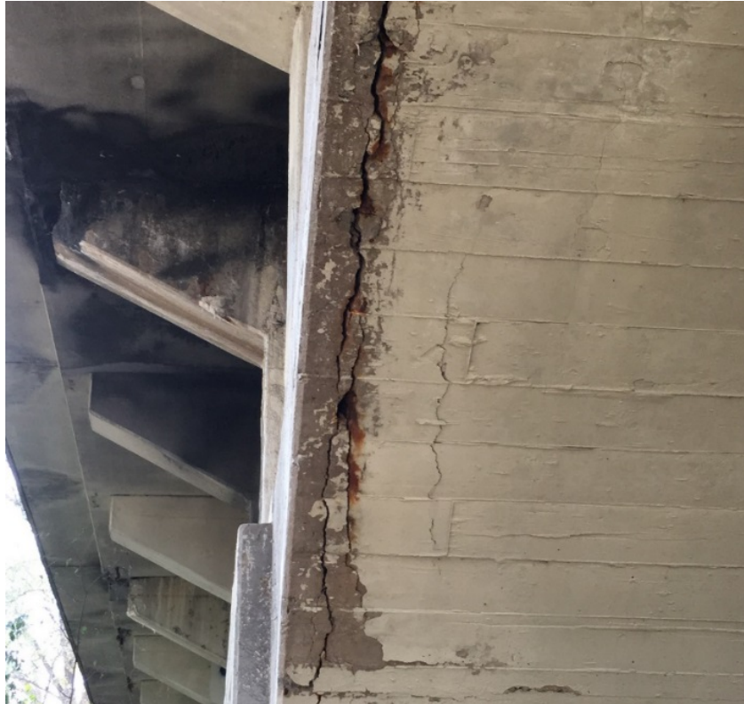
Figure 3: Cracks and Concrete Spalling on Arch Rib
