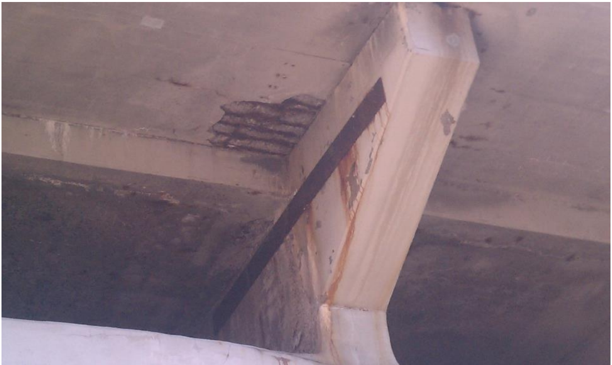
Figure 7: Spall on Deck, Spandrel Column Bracket with Strap Plate
