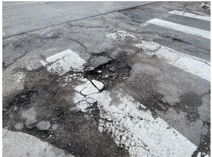
Degraded pavement in the crosswalk of 5 th Ave NE on the east side of Marshall St NE.
