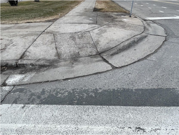
Aging pedestrian ramp without truncated domes, 8 th Ave NE intersection.
