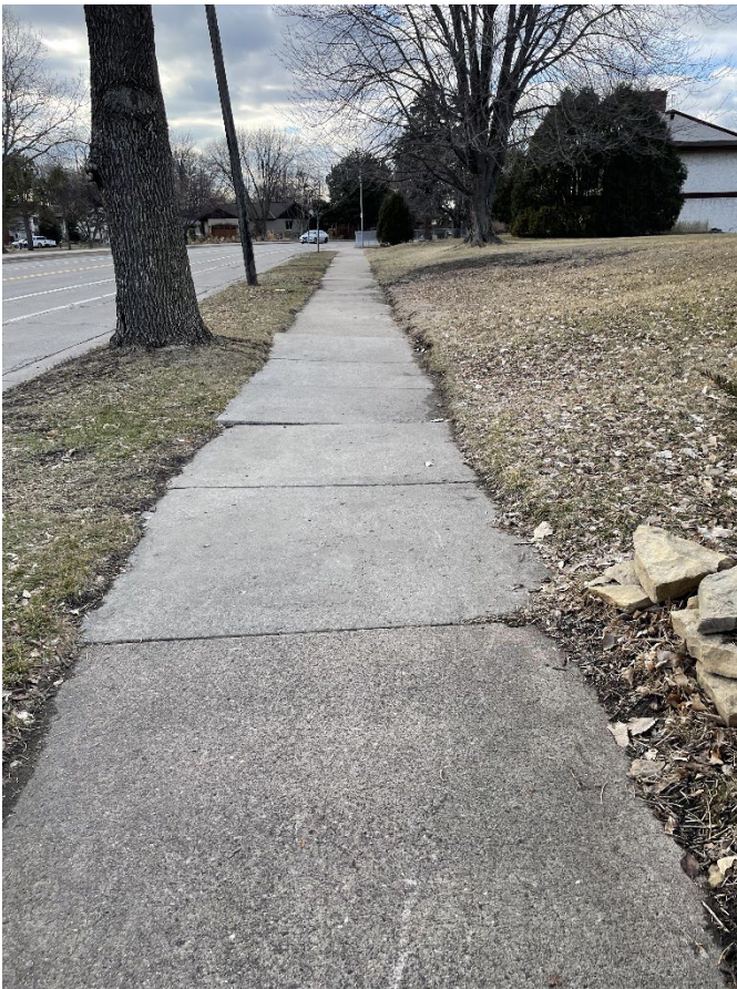
Uneven and aging concrete sidewalks, east side of Marshall St NE north of 8 th Ave NE.
