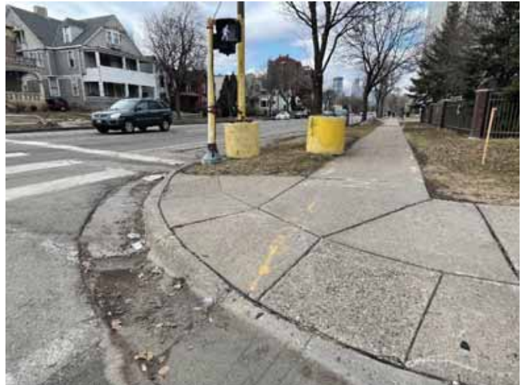
Lack of truncated domes and aging pedestrian ramps, 27 th and Park Ave intersection.
