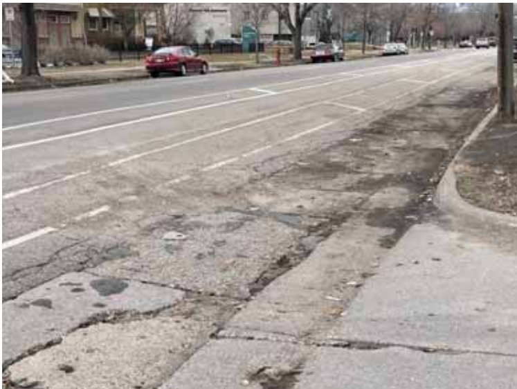
Cracked pavement assets and fading paint for on-street bicycle facilities on Park Ave.
