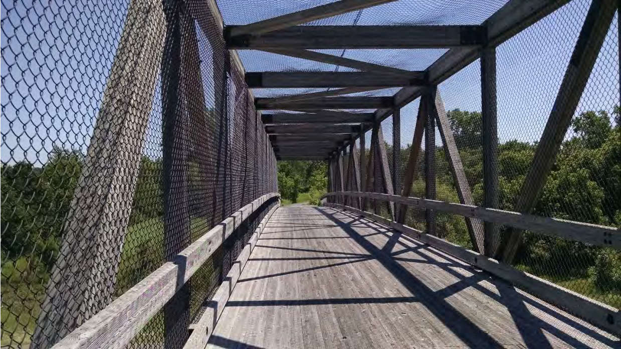
Rush Creek Trail – View from US Hwy 169 bridge west of the project area looking northeast.
