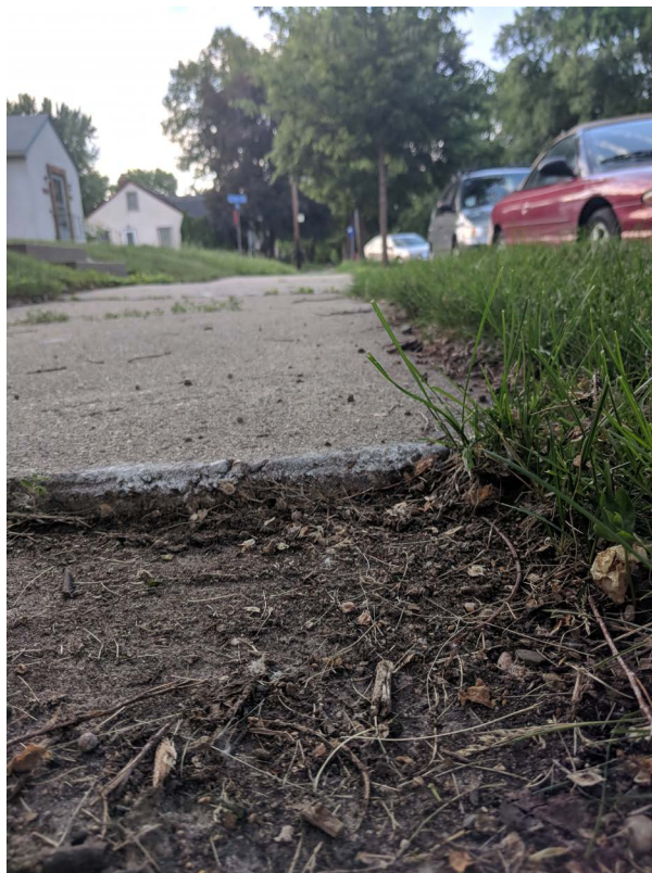
Figure 3-16: Vertical fault due to a settled sidewalk panel
