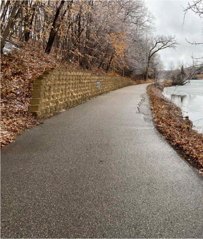
Paved trail segment, showing erosion at right
