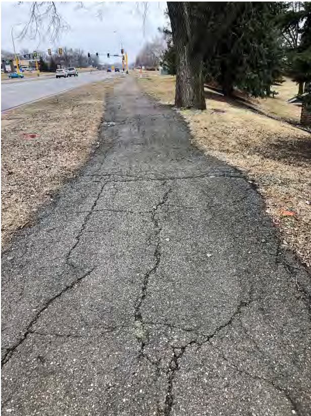
Fig 1. W 94 th to W 98 th Street, West side –Examples of deteriorated subgrade and pavement
