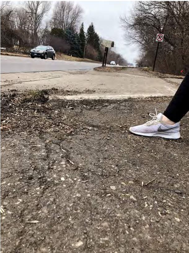
Fig 7. W 102 nd to Old Shakopee Road, East side – Example of ADA concerns with holes and driveway transitions
