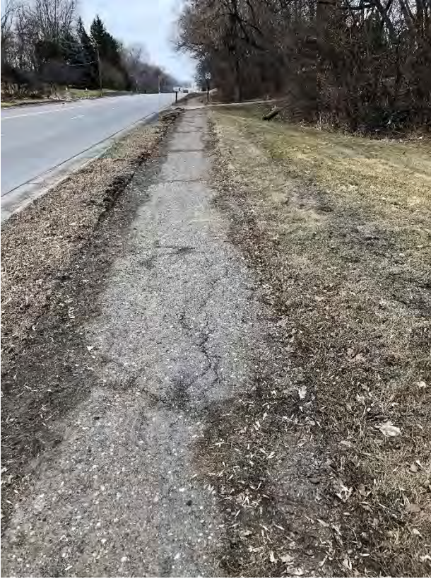
Fig 6. W 102 nd to Old Shakopee Road, East side –Example of deteriorated pavement and subgrade, narrow boulevard
