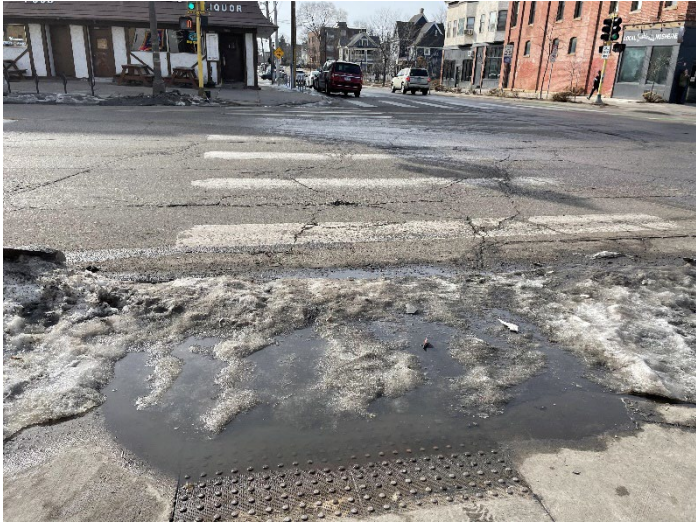
Even where truncated zones are present, ice and snow, as shown above at the 26 th St. intersection, pool at crossings due to drainage issues, creating barriers to accessibility.
