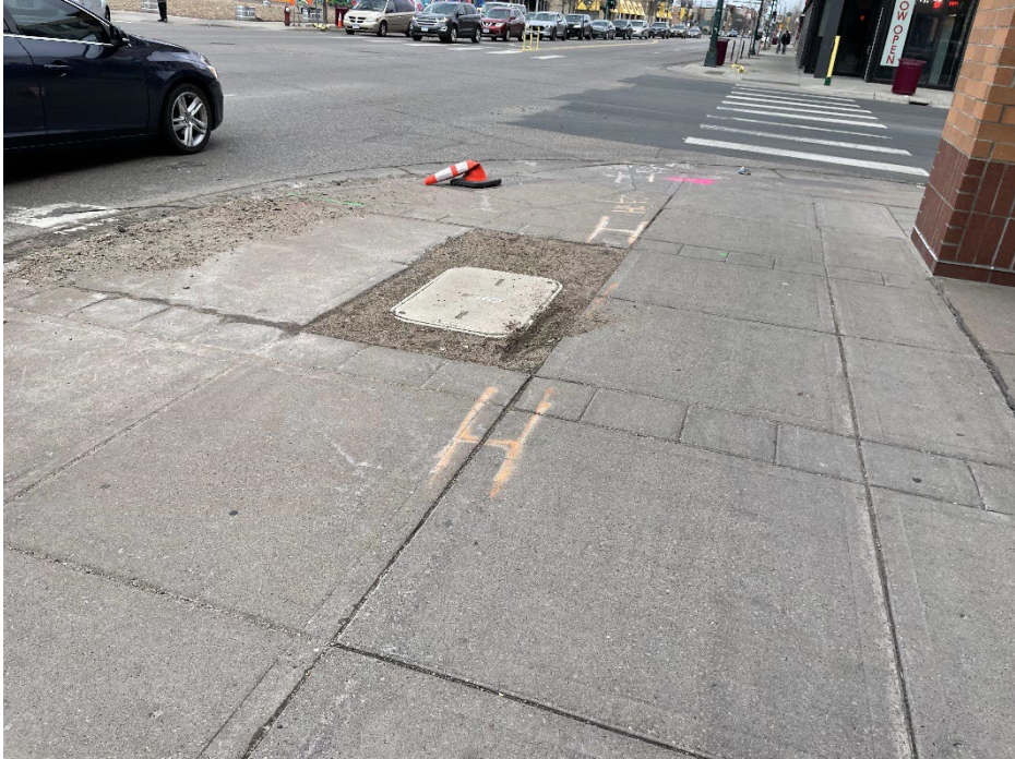
(Left) Sidewalk deficiencies such as this pose a barrier for future first and last mile transit connections for the Metro Transit B Line.
