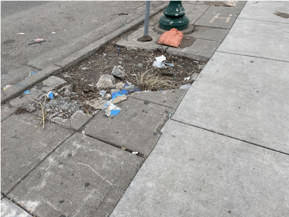
(Left) Sidewalk assets will be evaluated to address significant defects, such as this hole between Park and Portland Ave on Lake St.
