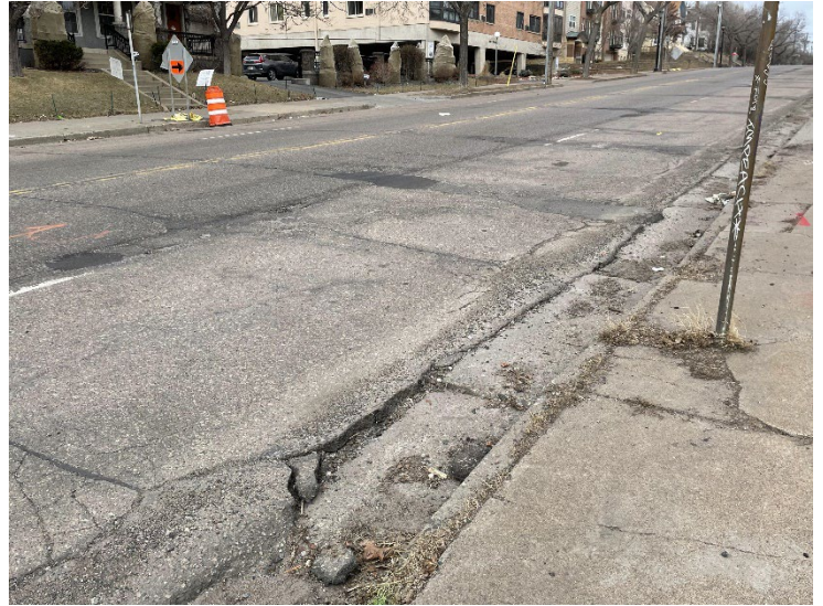
Many sections of the existing roadway, sidewalk and gutter pan are experiencing significant cracking and are in generally poor condition, as demonstrated above.
