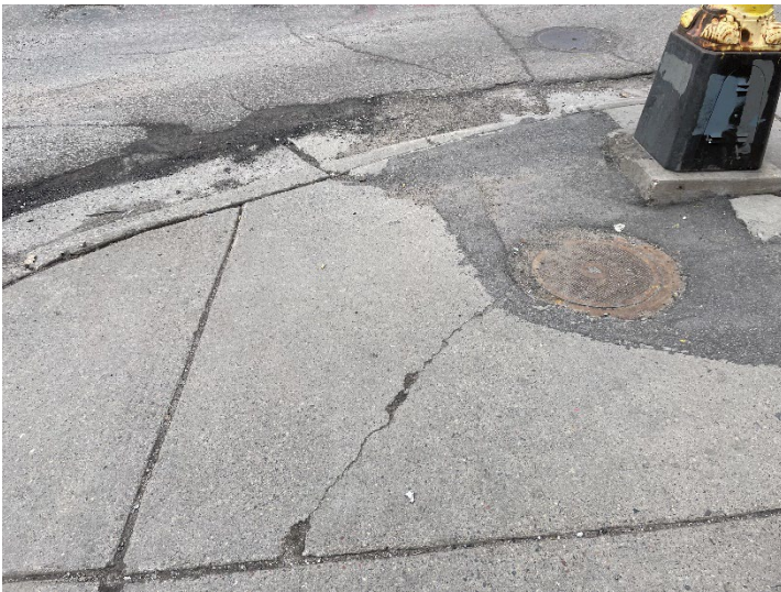
Three out of four quadrants at the Lyndale Ave and Franklin Ave intersection have older pedestrian ramps which are missing truncated domes. The signal at this intersection is 60 years old and is past its useful functional life.
