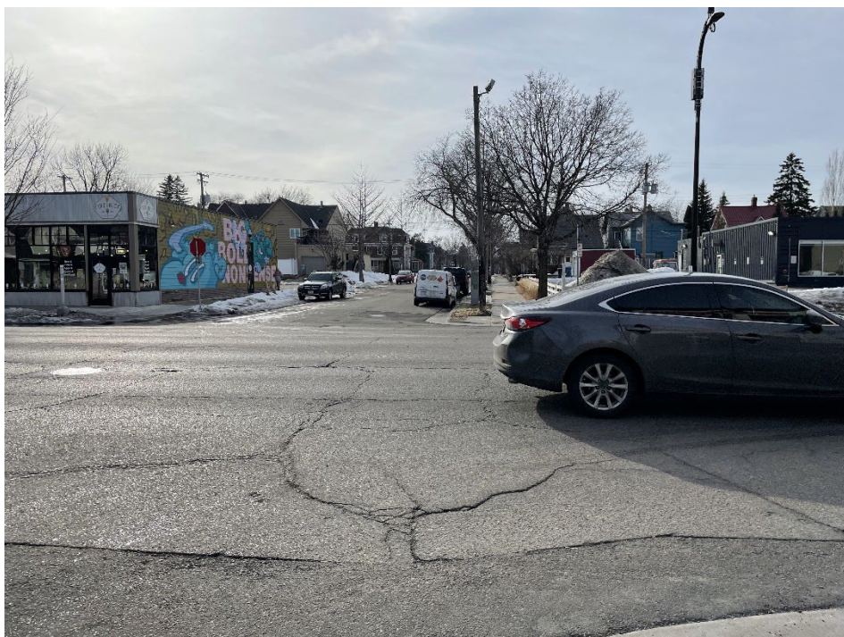
(Left) The intersection of 27 th and Lyndale Ave, is a barrier to pedestrians and cyclists due to high speeds and long crossing distances. Throughout the corridor, much of the roadway is experiencing significant cracking and pavement markings are worn.
