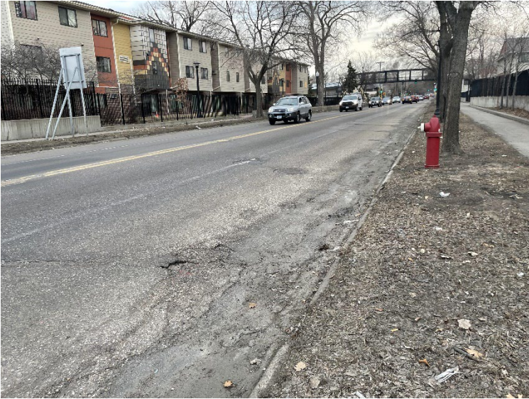
Existing roadway assets are past their useful life. As shown above, the outside lanes of Cedar Ave were transformed into parking lanes due to degrading pavement quality.
