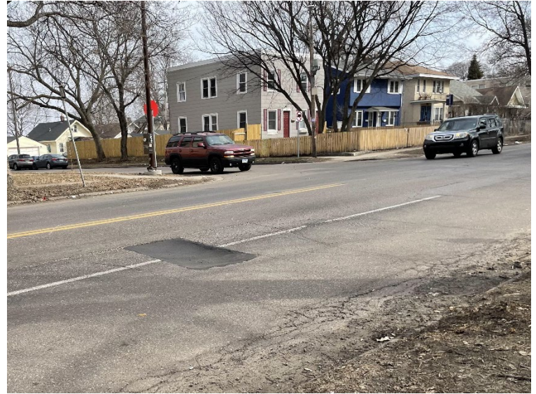
Pavement maintenance activities, such as the patch shown above, are no longer cost efficient for extending the useful life of the roadway.
