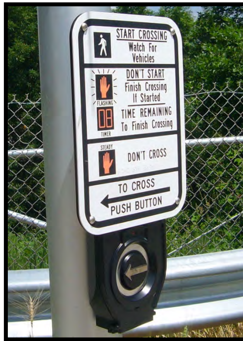
Figure C-5 Traffic Signal Pedestrian Phase
