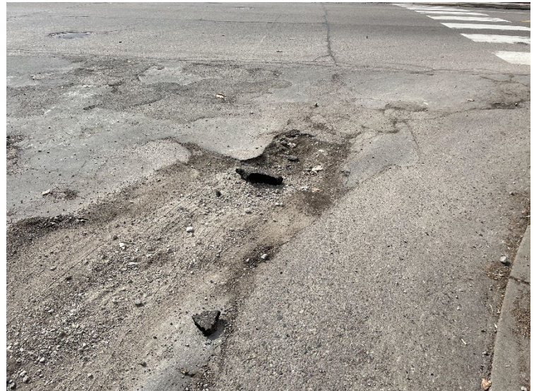
Degraded pavement assets obstructing pedestrian crossings at 74 th St.
