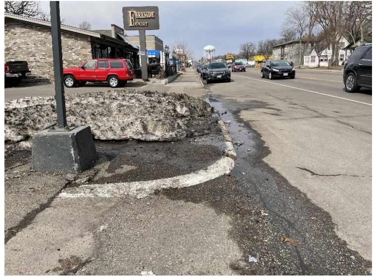
The corridor has significant sidewalk deficiencies, including this obstruction of snow and missing pedestrian ramp looking north at 68 th St.
