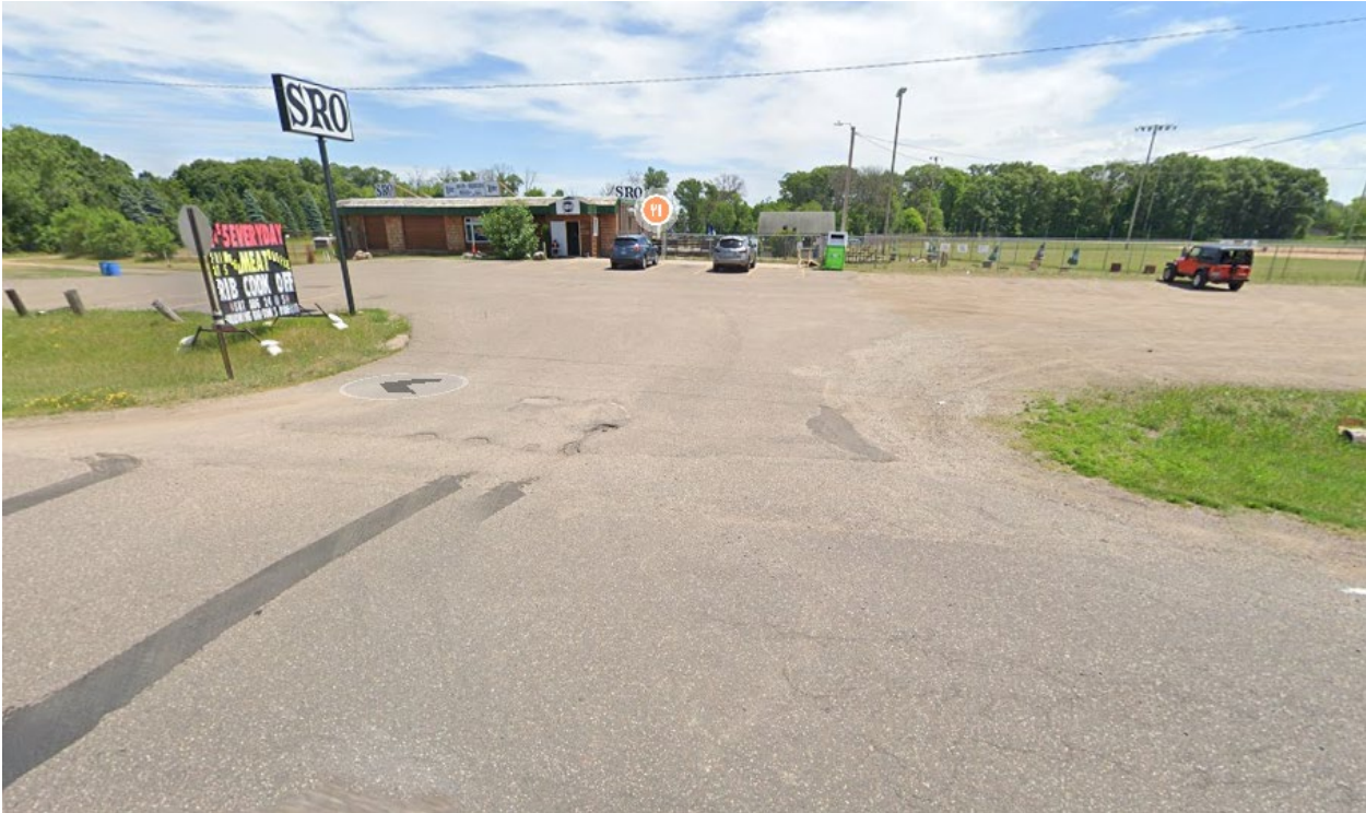
Inadequate driveway apron into commercial area.
