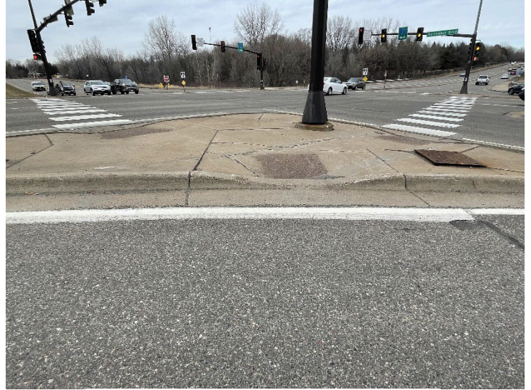
Aging pedestrian ramps lacking truncated domes at the southwest porkchop.
