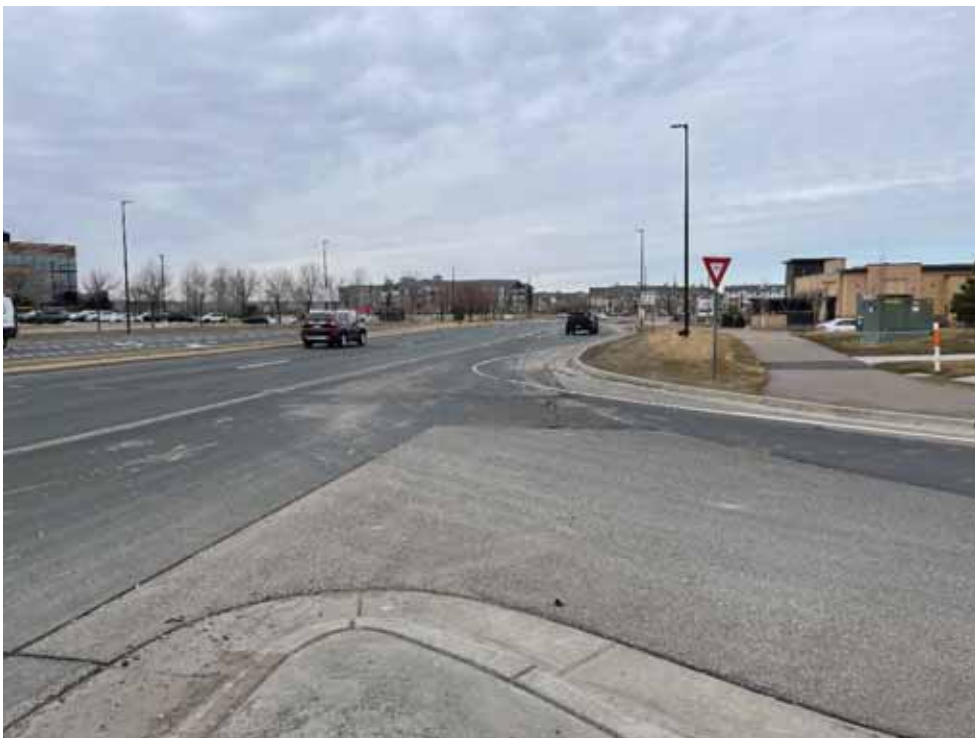
Eastbound free-right turn, demonstrating a lack of a marked crossing.
