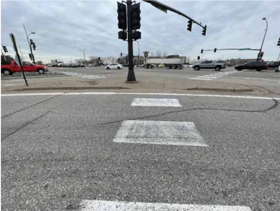
View of existing intersection, facing northwest at the southeast quadrant. Note the lack of truncated domes at the intersection porkchop.
