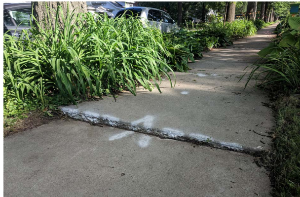
Figure 3-17: Vertical fault due to a heaved panel, likely from tree roots. This panel is marked for replacement through the city’s Defective and Hazardous Sidewalk Repair Program (SWK01).
