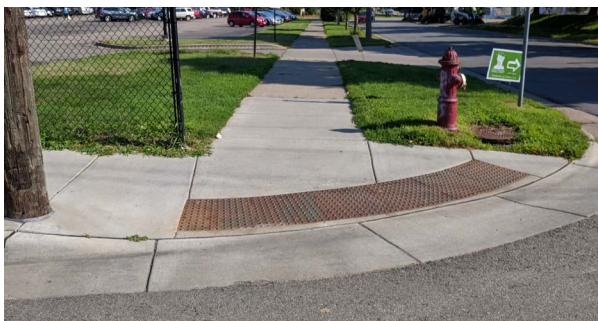
Figure 3-3: Fan Ramps or Depressed Corner Ramps provide one ramp to cross the street in either direction
