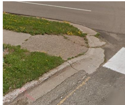
Example of a poor or non-compliant pedestrian ramp
