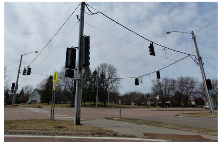
Existing Carver County Traffic Signal
