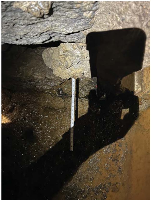
Under mining of the west storm outlet under culvert.
