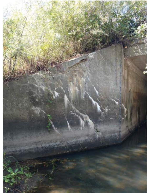
Large spall with efflorescence on side of bridge structure pictured above.
