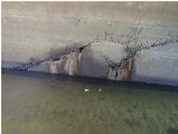
Culvert honeycomb leakage middle of south wall barrel with efflorescence requires repair.
