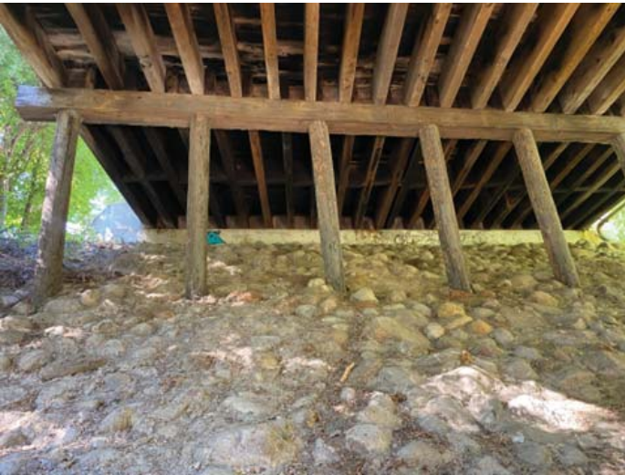
Side profile of the existing bridge, as viewed from the Luce Line State Trail from below.
