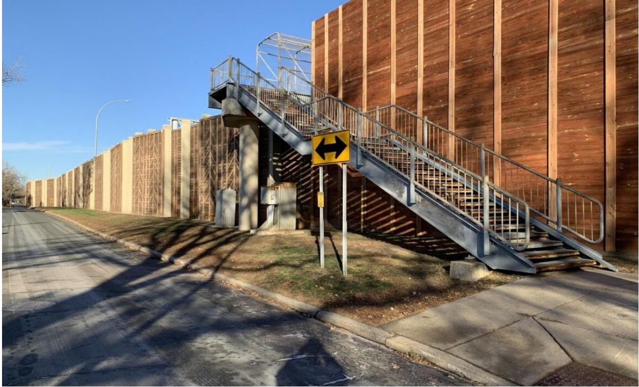
Photo 3: Stairs on the west side of existing Bridge #9888 over I-35W (Nov 2023). Photo Credit: City of Richfield
