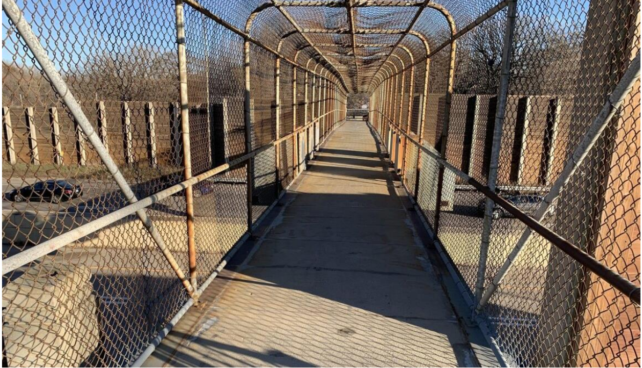
Photo 1: Cross section of existing Bridge #9888 over I-35W (Nov 2023). Photo Credit: City of Richfield
